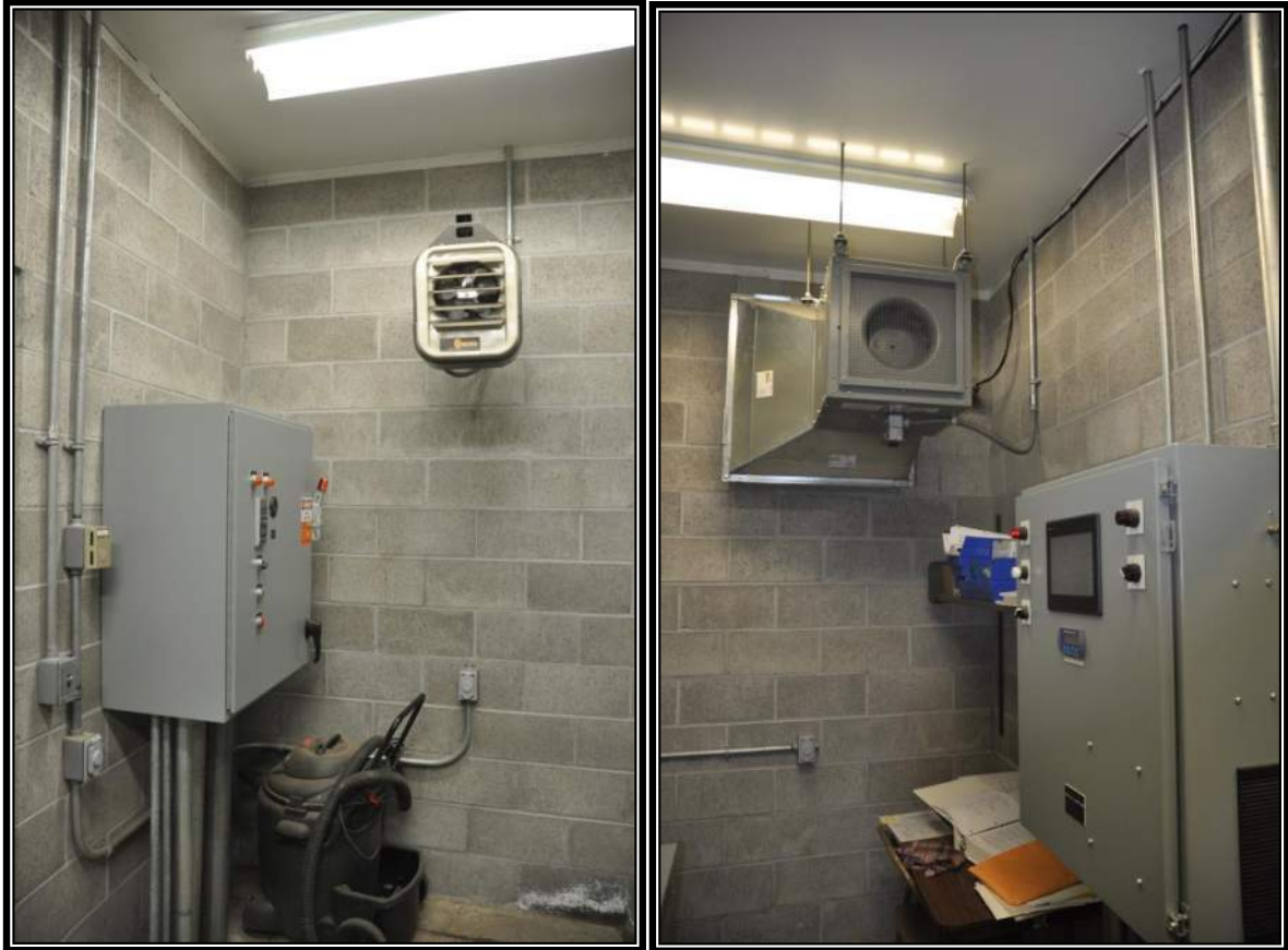
ASR Pump Station – Electrical Cabinets & Hanging HVAC Equipment
