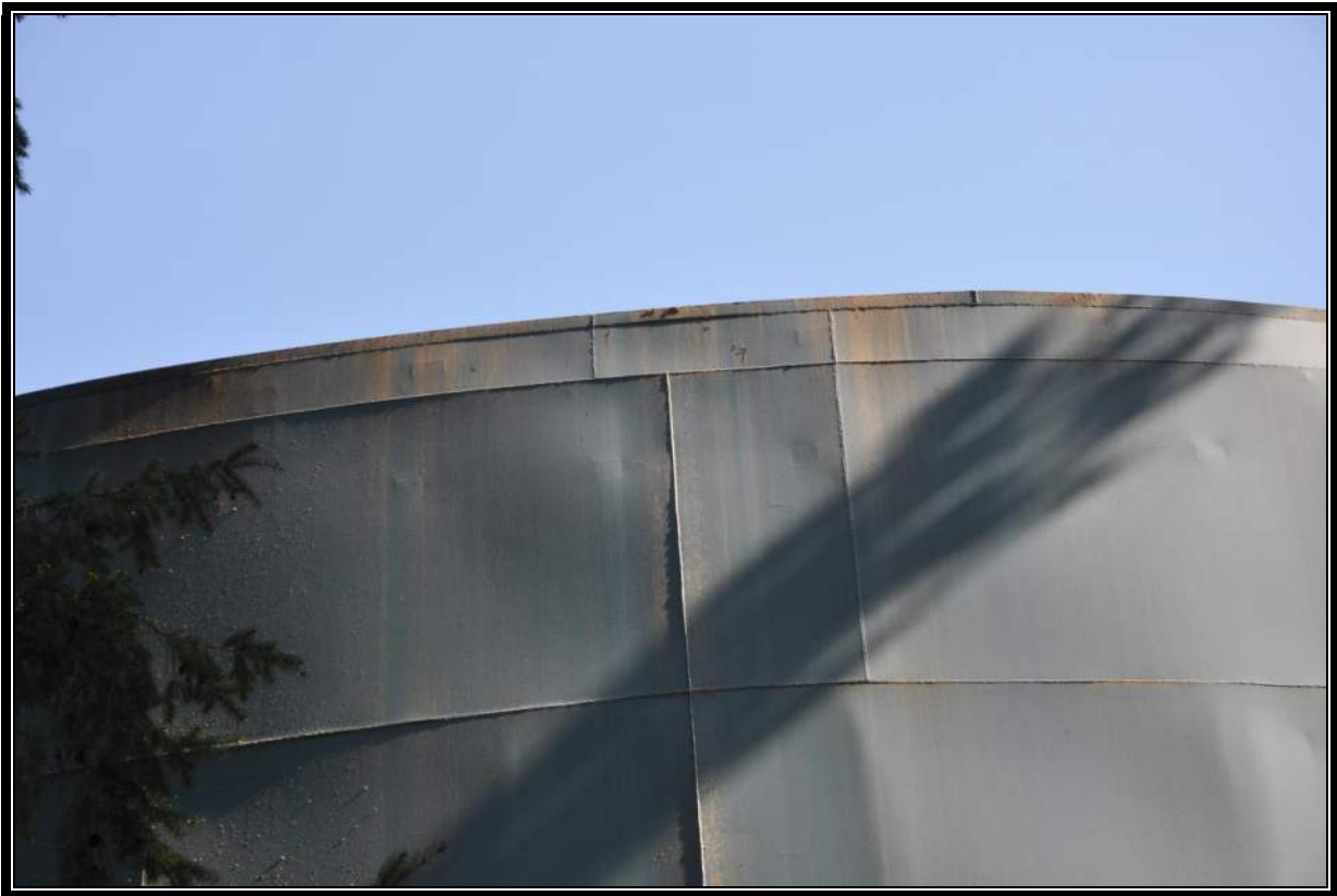
2.2 MG A1 Reservoir – Buckled Wall Shell Plates
