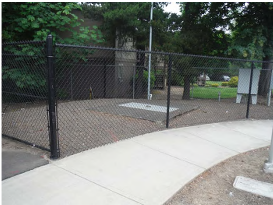
Photo 7: Boones Ferry Road Pump Station and Supply Control Valve (May 30, 2018).
