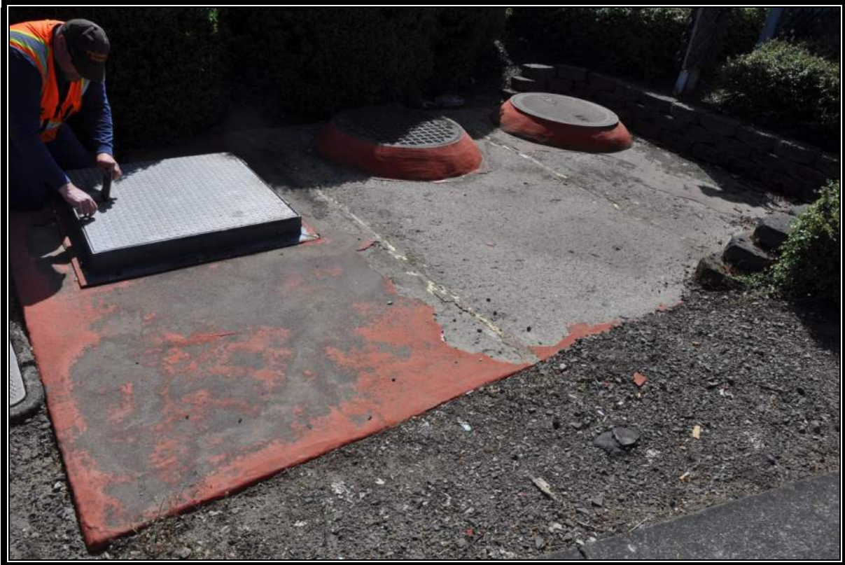
Martinazzi Pump Station
