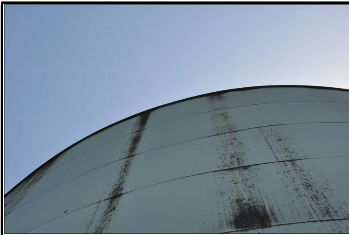
2.2 MG B2 Reservoir – Wall Shell Plates
