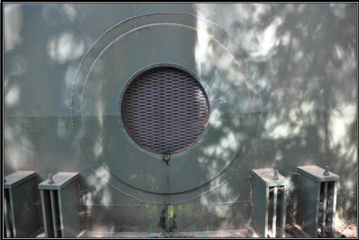
2.2 MG A1 Reservoir – Overflow Discharge
