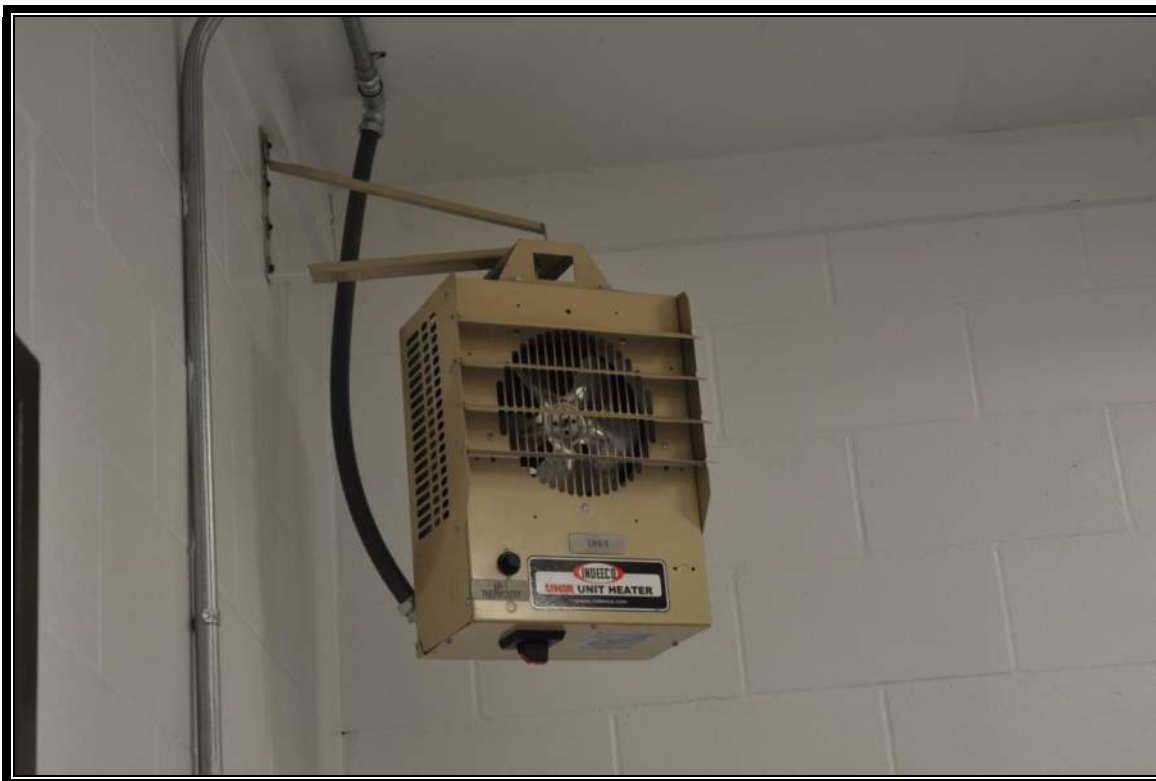
C Level Norwood Pump Station – HVAC Equipment with Limited Lateral Strength
