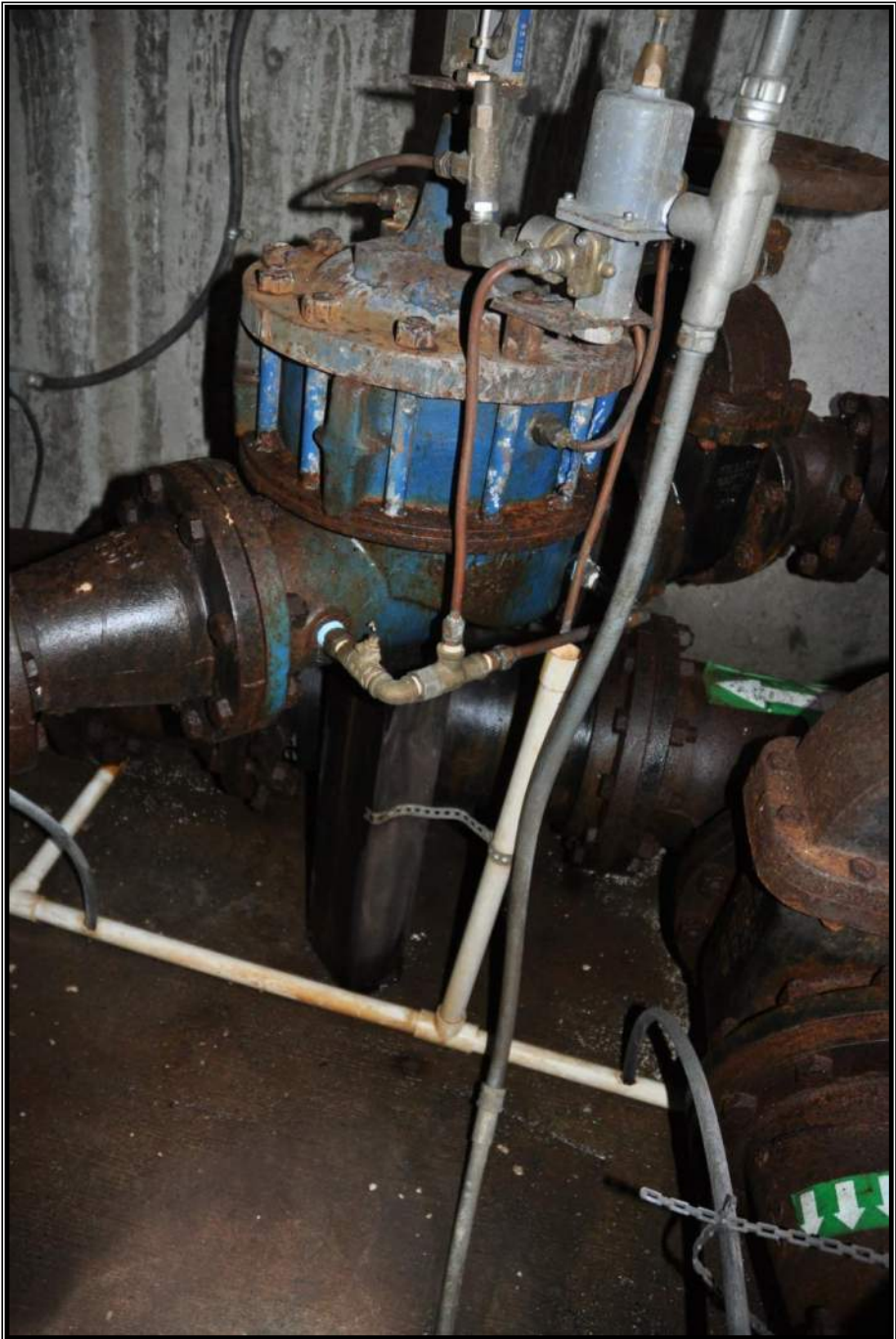
Martinazzi Pump Station – Outdated Pipe Bracing
