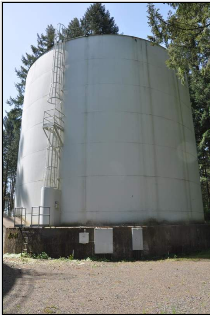
0.8 MG C1 Reservoir
