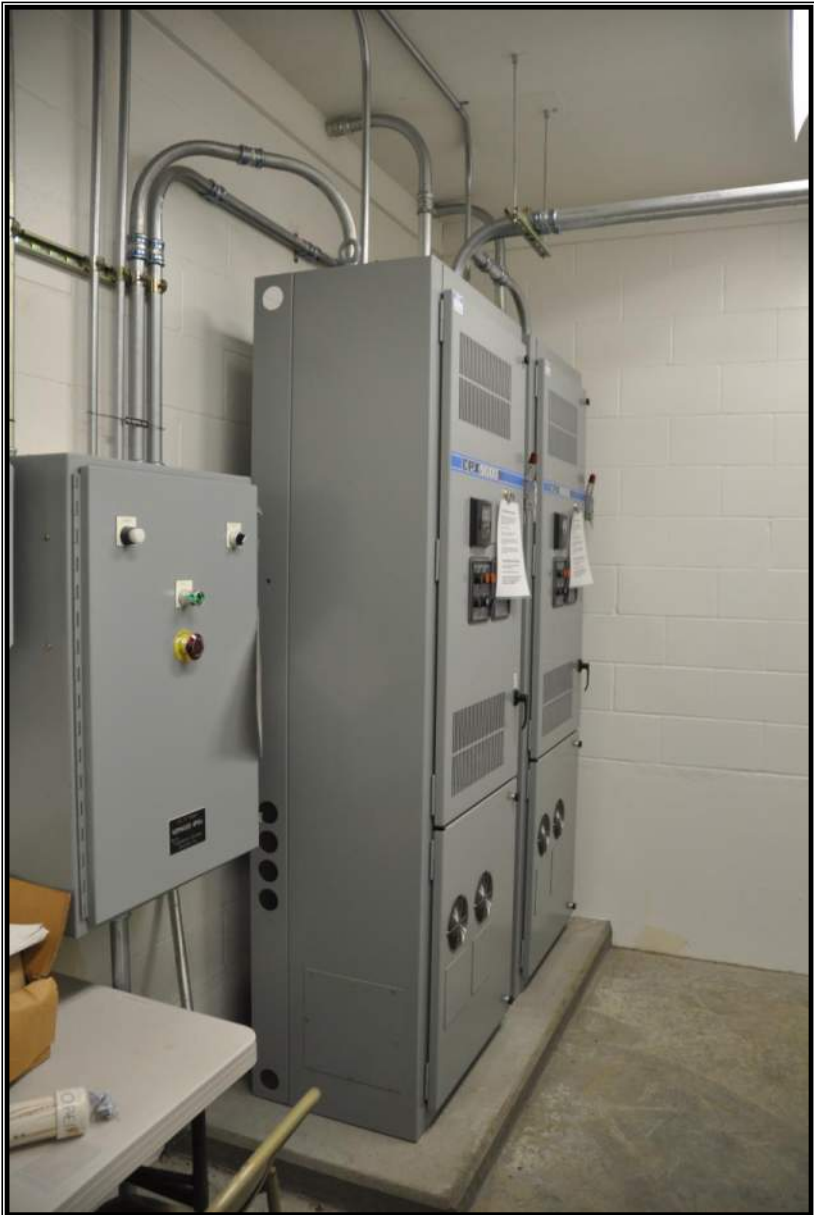
C Level Norwood Pump Station – Electrical Cabinets, Verify/Add Lateral Bracing
