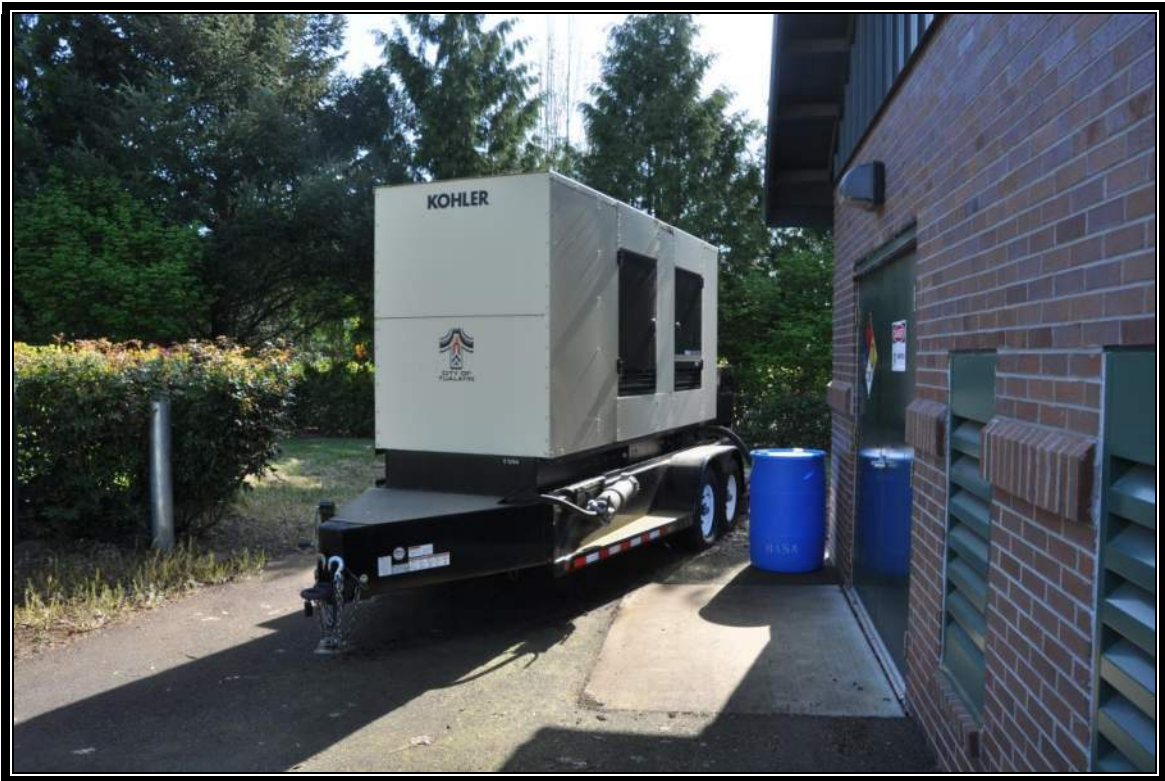
ASR Pump Station – Temporary Generator
