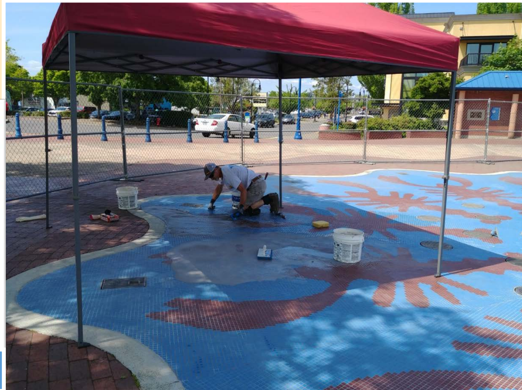
TUALATIN COMMONS SPLASH PAD SURFACE EMERGENCY REPAIR
