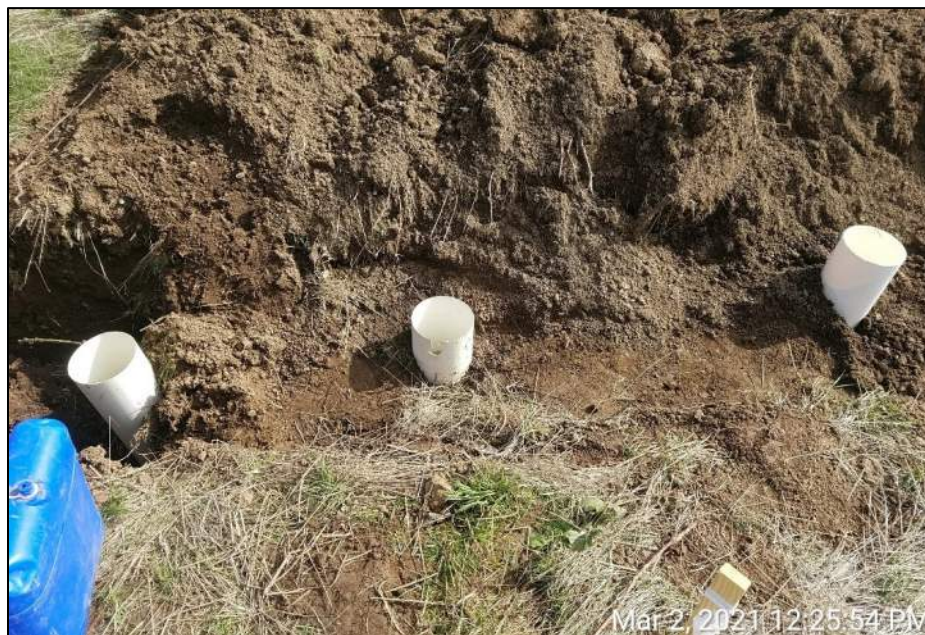
Photo 7: Backfilling around the 3 standpipes in the test pit trench at one of the infiltration test locations prior to conducting the infiltration testing.
