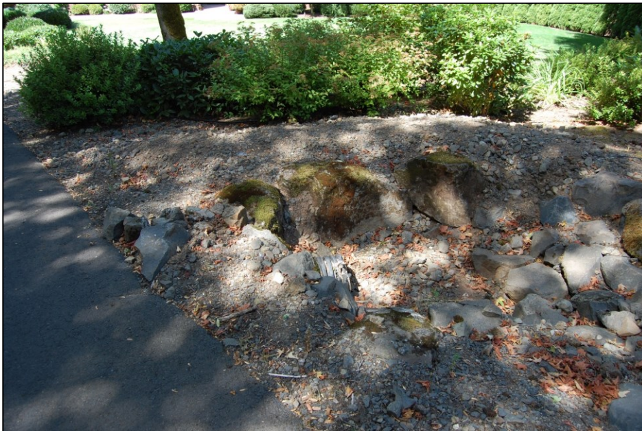
Photo A3d. This photo of the westernmost base of the ditch was taken on August 19, 2016 and looks generally west toward the Lucini house. Shown the basin where stormwater collects and is routed into the entrance of the 12-inch corrugated plastic pipe (CPP), which is visible in the center of the photo. This pipe entrance allows flows to go south into the driveway culvert. Although a reversed view, this photo corresponds to the flood location in Photo A2c of the previous Appendix A2.
