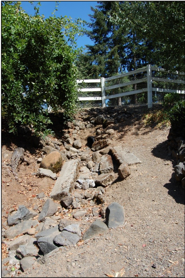
Photo A3a. This photo of the Lucini property ditch was taken on August 19, 2016 and looks generally northeast up the slope to the pipe end exiting from the County's road project. This photo shows the continuing effects of erosion with the ditch spreading east and west into the embankment where bare soil and tree roots are exposed. To slow flows the owner has placed riprap and concrete block in the ditch to reduce stormwater flow velocities that continue to erode the channel requiring ongoing repairs. This photo corresponds to the flood location in photo A2a of the previous Appendix A2, which shows high velocity storm flows into the Lucini property.
