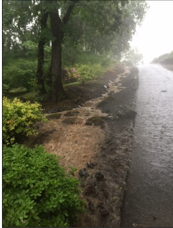
Photo A2c. The junction for the ditch and driveway pipe are overwhelmed and flood waters drain into the front yard toward the house (5-18-15).
