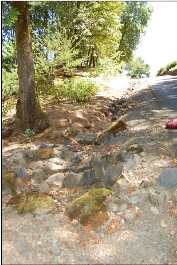
Photo A3c. This photo of the Lucini property ditch was taken on August 19, 2016 and looks generally northeast up the slope. This photo shows the continuing effects of erosion with the ditch spreading north into the embankment where bare soil and tree roots are exposed. To slow flows the owner has placed riprap in the ditch to reduce stormwater flow velocities that continue to erode the channel requiring ongoing repairs. This photo corresponds to the flood location in Photo A2c of the previous Appendix A2. The entrance to the 12-inch driveway culvert, which carries stormflows to the right (to the south), is hidden from view by the large rock at the bottom of the photo. See the next photo (A3d) for a view of the entrance to the driveway culvert).
