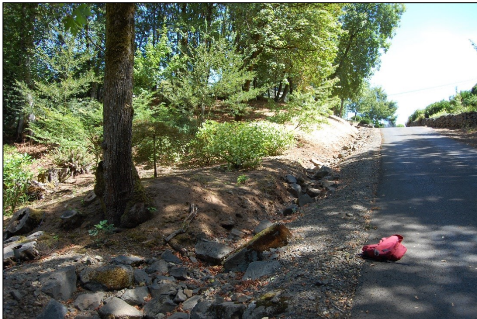
Photo A3b. This photo of the Lucini property ditch was taken on August 19, 2016 and looks generally east up the slope of the driveway. This photo shows the continuing effects of erosion with the ditch spreading south toward the driveway, and north into the embankment where bare soil and tree roots are exposed. To slow flows and reduce erosion, the owner has placed riprap in the ditch and gravel next to the driveway. However, very high stormwater velocities continue to erode the channel requiring ongoing repairs.
