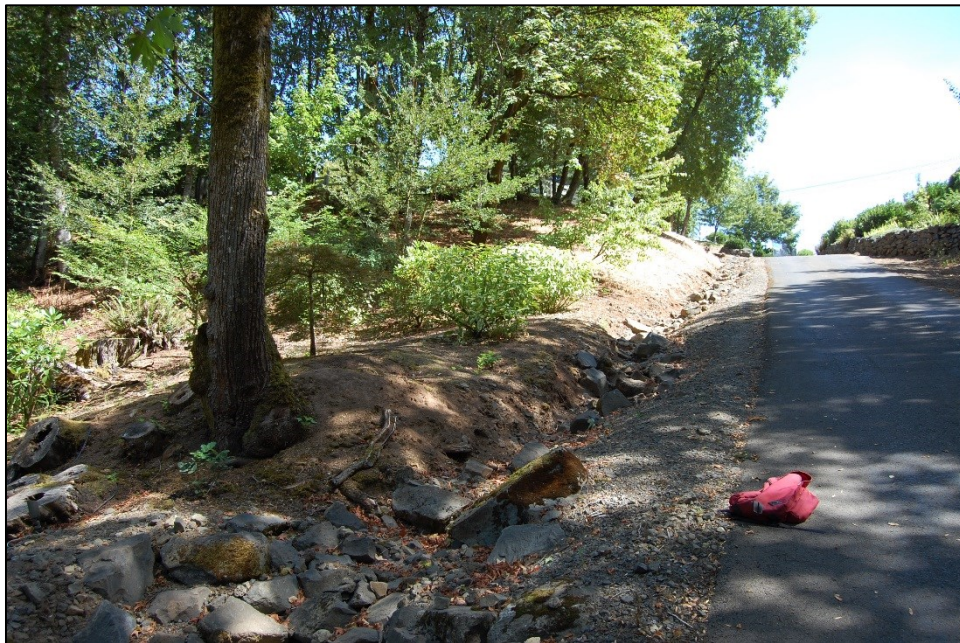
Photo A3b. This photo of the Lucini property ditch was taken on August 19, 2016 and looks generally east up the slope of the driveway. This photo shows the continuing effects of erosion with the ditch spreading south toward the driveway, and north into the embankment where bare soil and tree roots are exposed. To slow flows and reduce erosion, the owner has placed riprap in the ditch and gravel next to the driveway. However, very high stormwater velocities continue to erode the channel requiring ongoing repairs.
