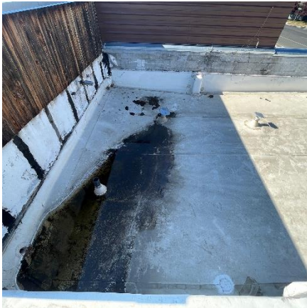
Roof Ponding and Clogged Drain
