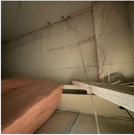
2x4 Stud Wall Adjacent to CMU Block Stud Walls Joined Above Drop Ceiling
