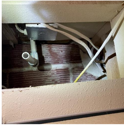
PVC Pipe Termination Near Restroom Undetermined Use
