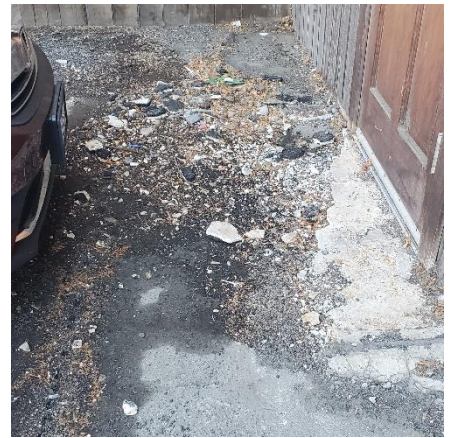
Degradation of North Entry Pavement
