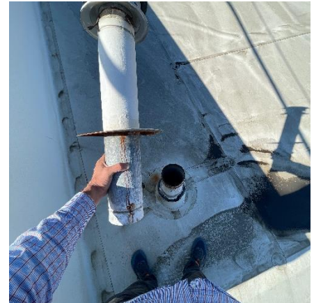
Detached HVAC Vent Assembly
