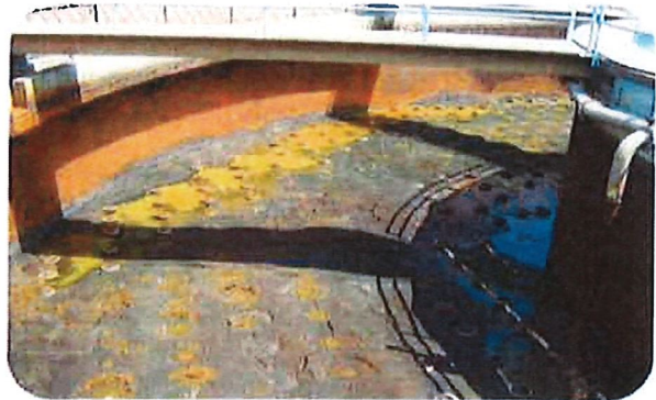
Grit Deposition in Process Basins
