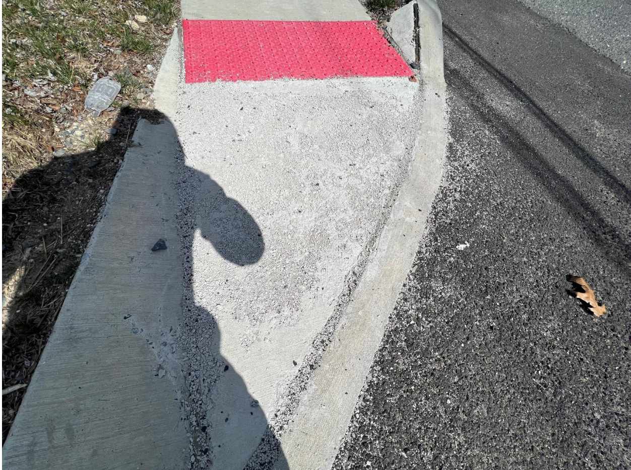
Attachment #1: Concrete spalling on ADA ramp.
