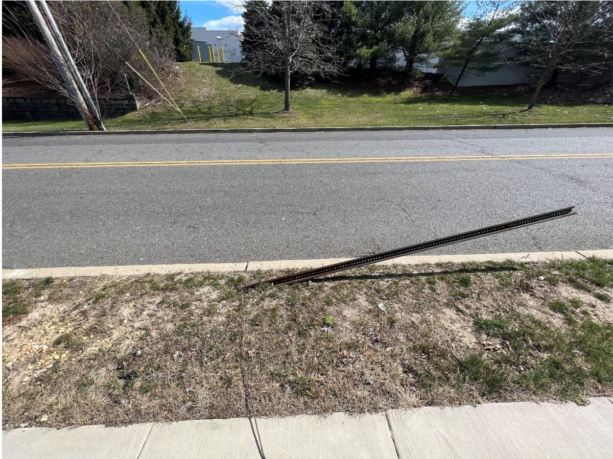
Attachment #2: Pole to be removed.
