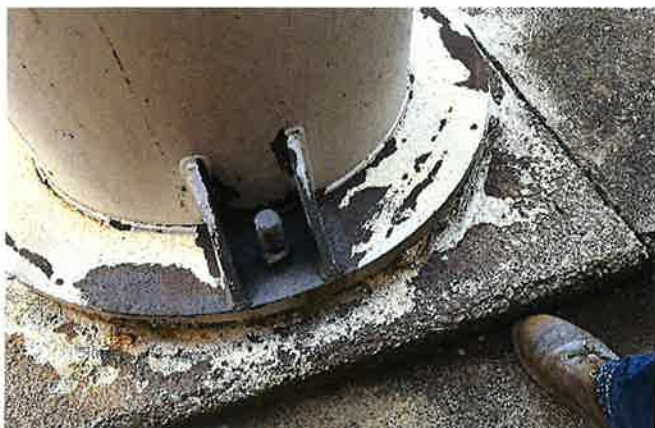
SANDBLASTED CORROSION ON/AROUND ANCHOR BOLTS
