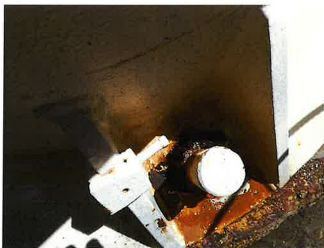
GENERAL CORROSION W/UNDERCUTTING
