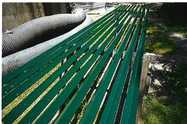
METAL BARS FOR T-MOBIL EQUIPMENT
