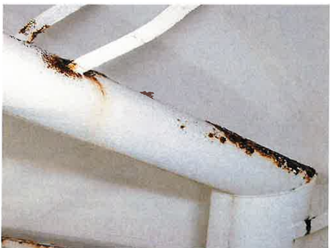
OVERFLOW PIPE CORROSION
