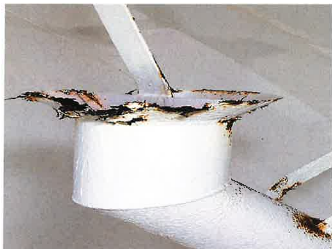
TOP OF OVERFLOW PIPE CORROSION
