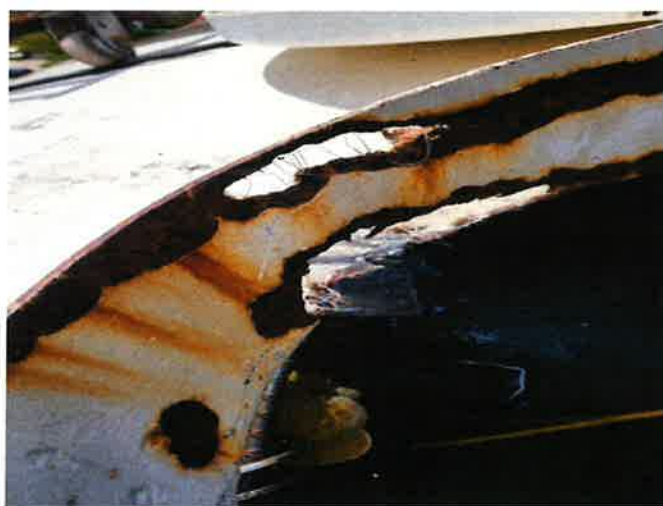
ROOF PLATE AND COLLAR SEVERELY CORRODED
