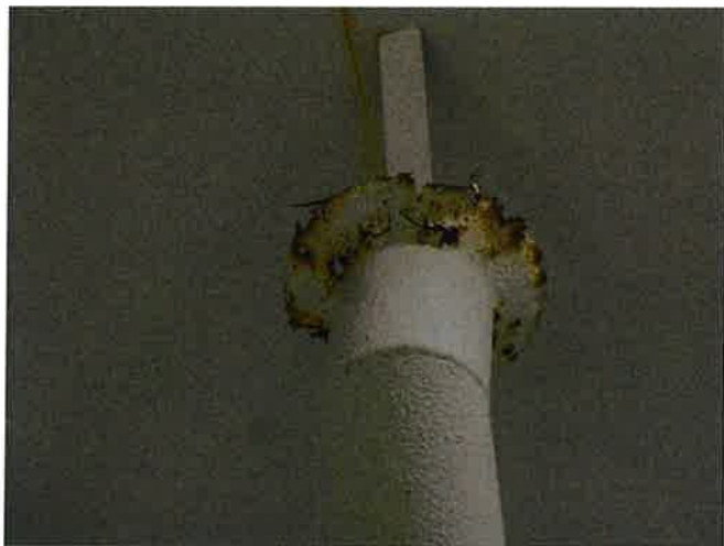
OVERFLOW TOP HAT EXCESSIVE CORROSION
