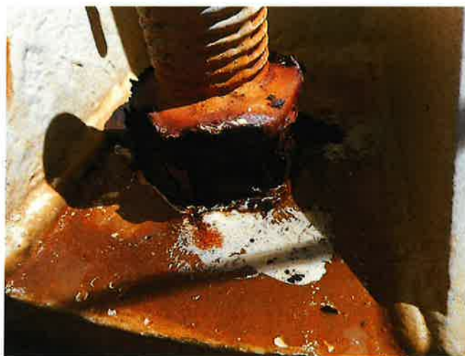
GENERAL CORROSION W/UNDERCUTTING
