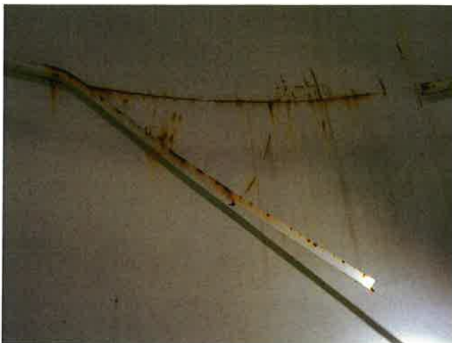
STIFFENER RING CORRODED AND DETACHED FROM TANK
