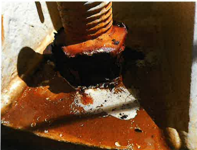
GENERAL CORROSION W/UNDERCUTTING
