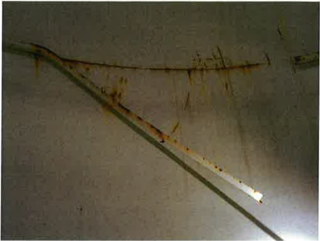
STIFFENER RING CORRODED AND DETACHED FROM TANK
