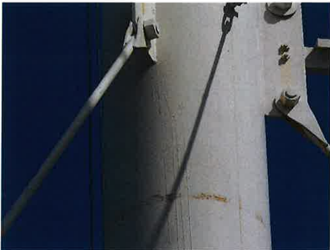
RUNS IN COATING PREVIOUS APPLICATION
