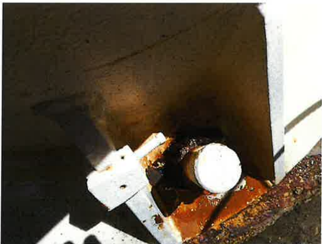
GENERAL CORROSION W/UNDERCUTTING
