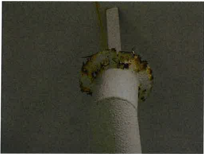
OVERFLOW TOP HAT EXCESSIVE CORROSION
