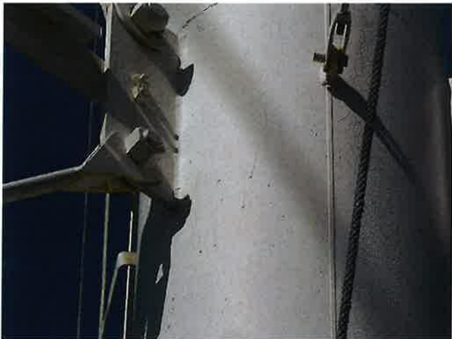
RUNS IN COATING PREVIOUS APPLICATION
