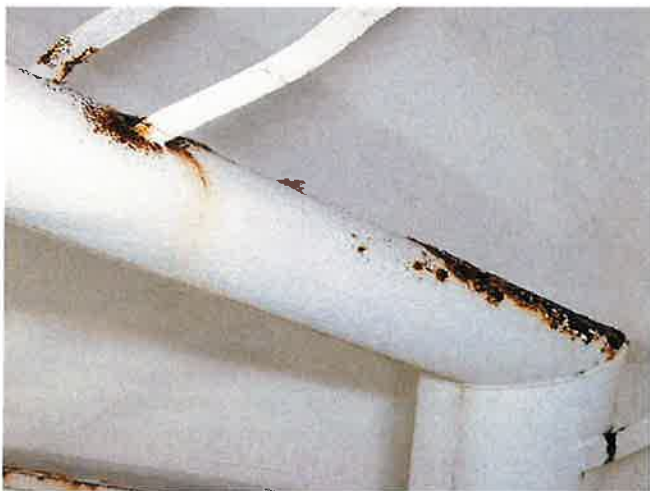
OVERFLOW PIPE CORROSION
