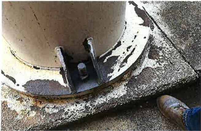
SANDBLASTED CORROSION ON/AROUND ANCHOR BOLTS
