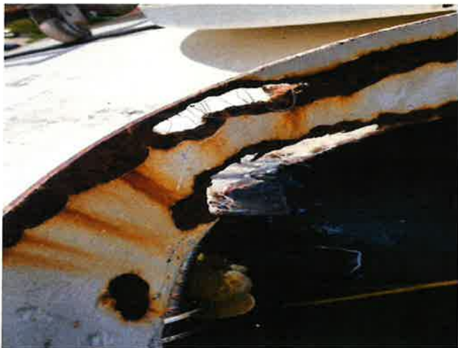
ROOF PLATE AND COLLAR SEVERELY CORRODED
