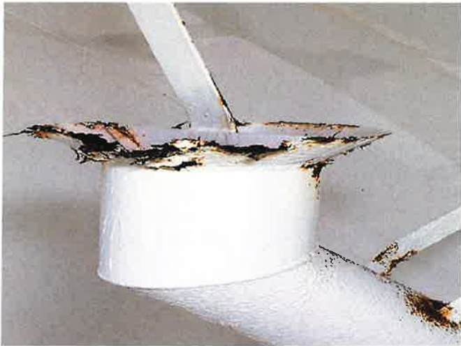
TOP OF OVERFLOW PIPE CORROSION
