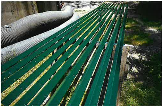
METAL BARS FOR T-MOBIL EQUIPMENT
