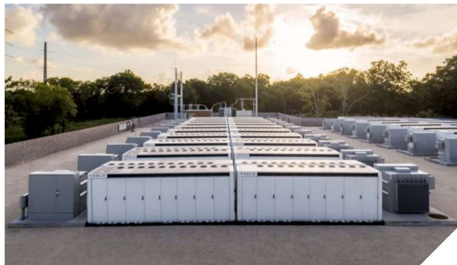
Tesla's Megapack stand-alone storage system.
