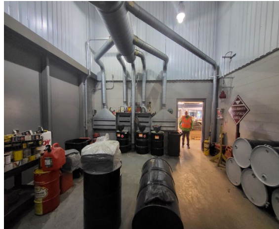
Figure 5-2. HazoHouse Bulking Room
