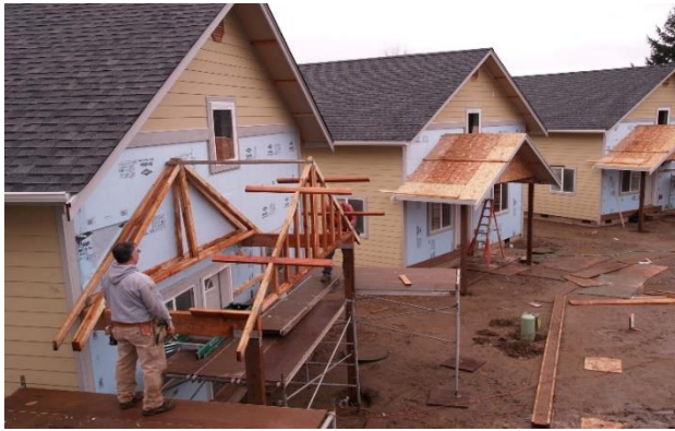
Figure 2 Thurston County funded Habitat for Humanity of South Sound to build five more houses for low-income first-time home-buyers in their Deyoe Vista Sub-division in Lacey. (Photo credit: Shanna Paxton Photography)
