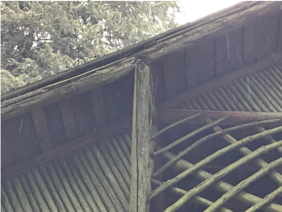
Picture 6 – dry rot damage
