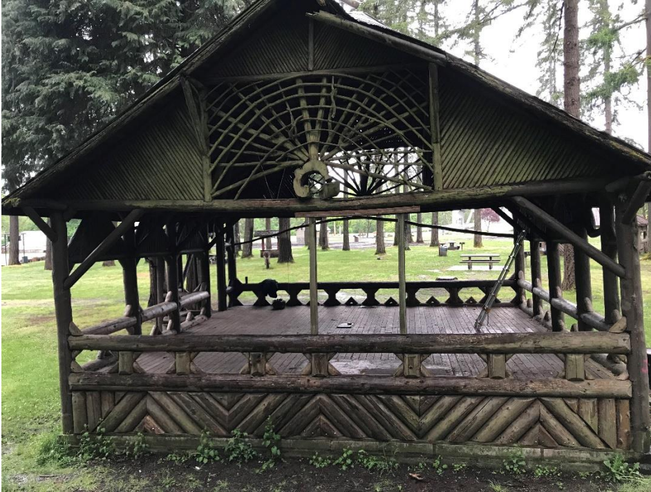
Picture 5 -south side tree damage and shoring
