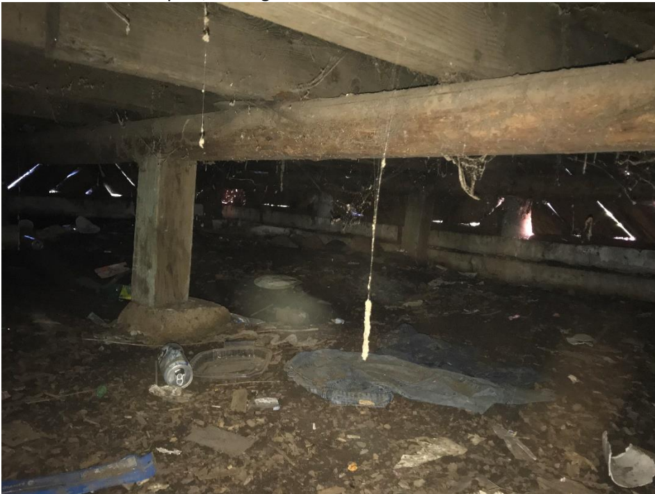
Picture 13 – shifted post/footing
