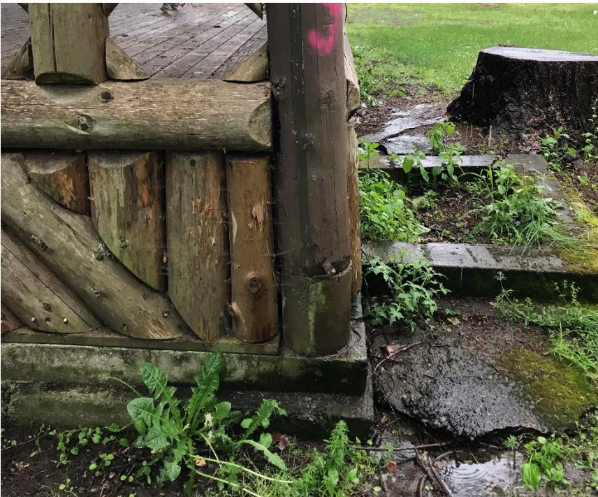
Picture 10 – foundation movement and stump
