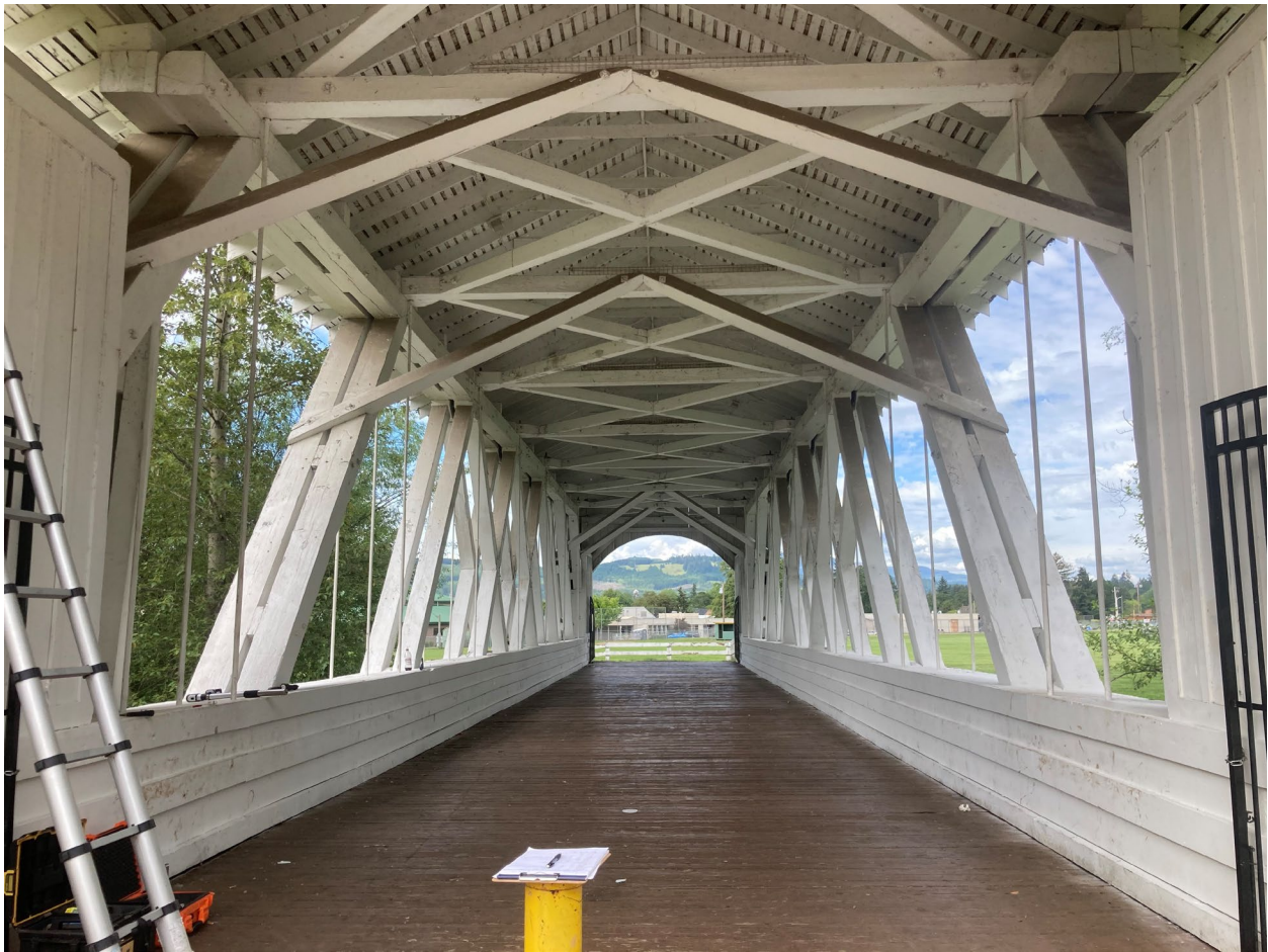
Figure 16 – Inside Paint condition
