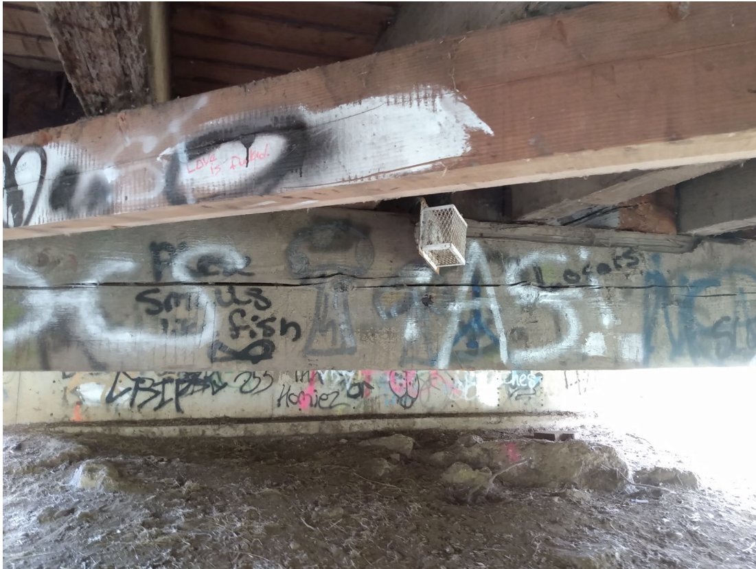
Figure 12 - Bent 2 scour – monitor scour after peak rainfall events.
