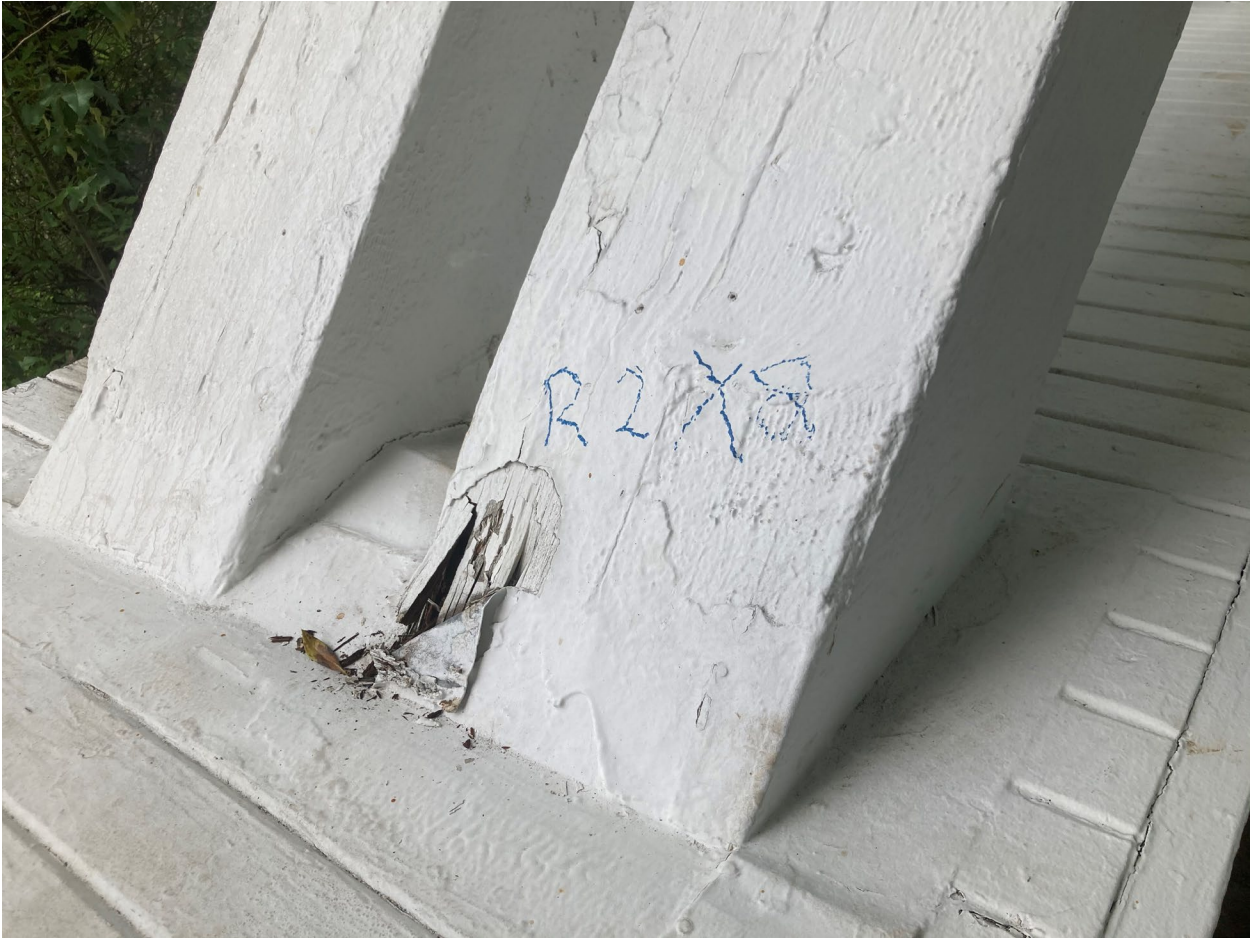
Figure 5 – Downstream L3U4 (right) 2” of minor decay
