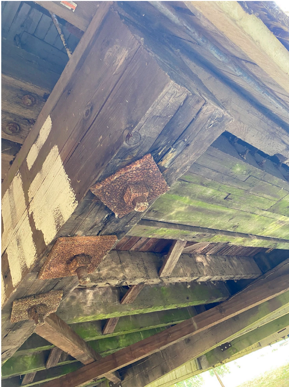
Figure 9 – Pitting on tie rod anchors
