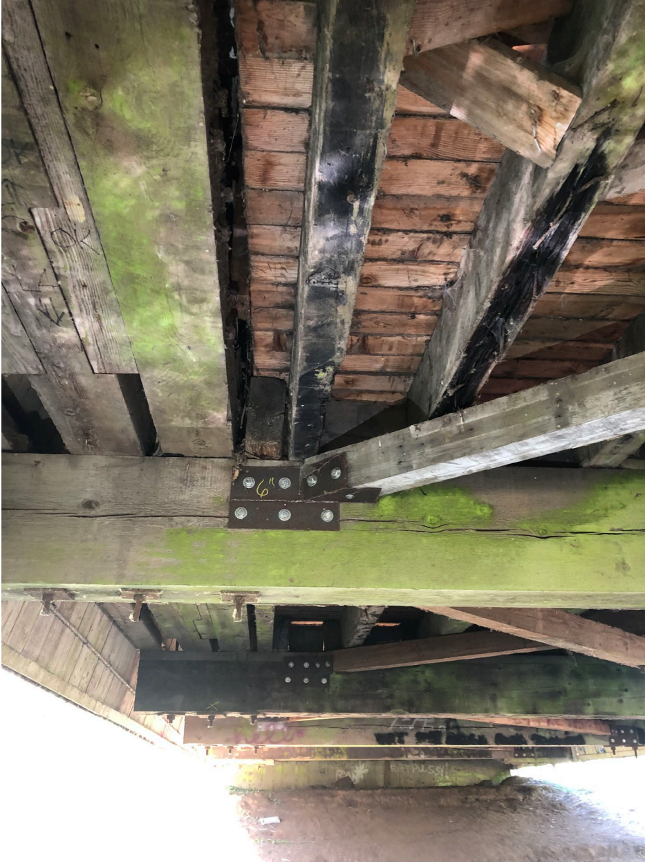
Figure 11 - Surface decay and fire damage to Bay 5 Stringers 7 & 8
