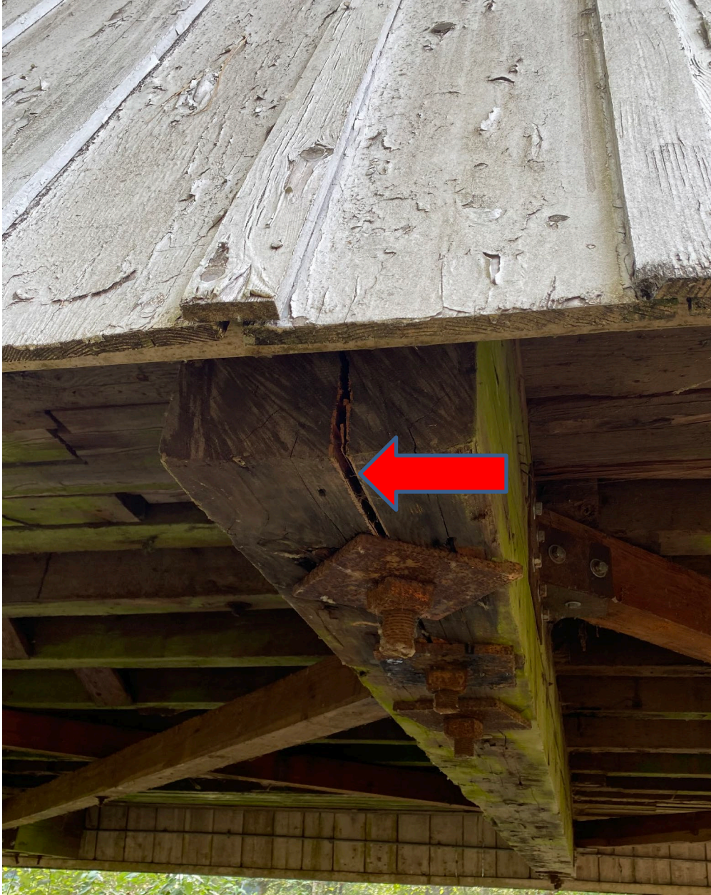
Figure 8 – Split at end of Floor Beam 3
