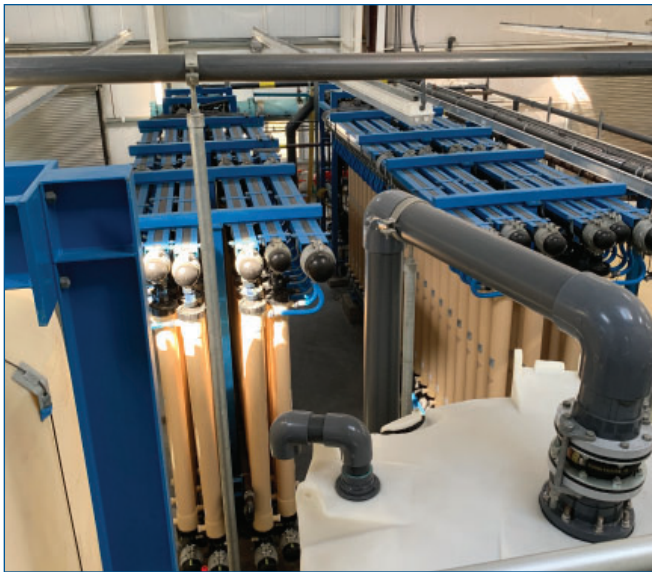
West Yost's team recently assisted the City of Cottage Grove in the design and construction of an expansion of the City's Row River membrane water treatment facility.
