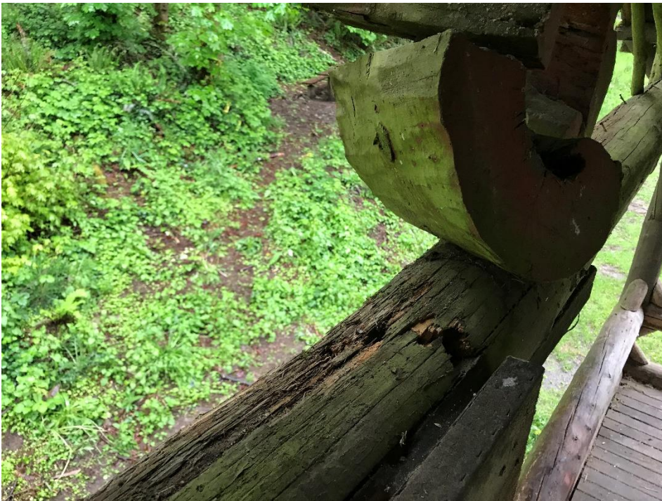
Picture 2 – Broken main member
