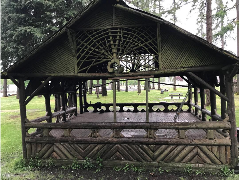
Picture 5 -south side tree damage and shoring
