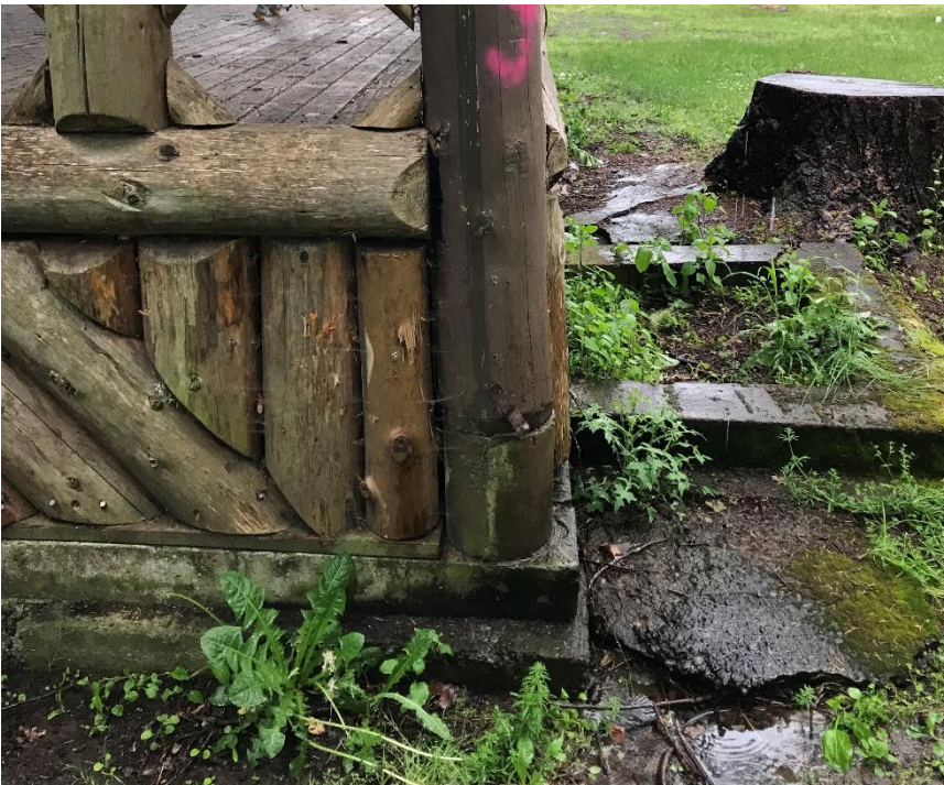
Picture 10 – foundation movement and stump
