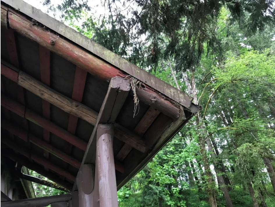
Picture 7 – dry rot damage
