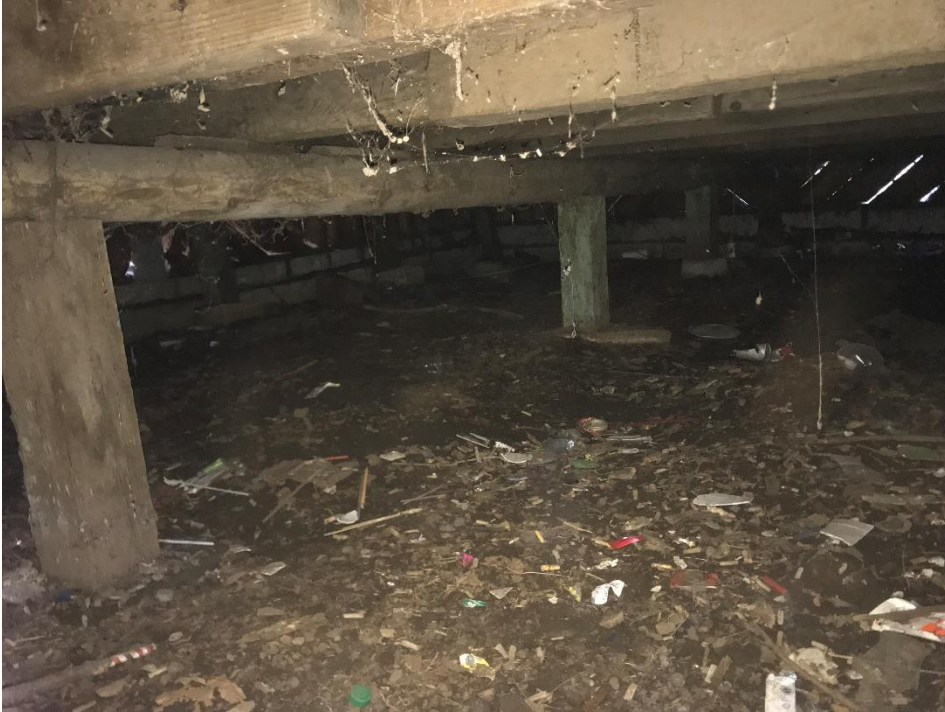
Picture 14 – shifted footings
