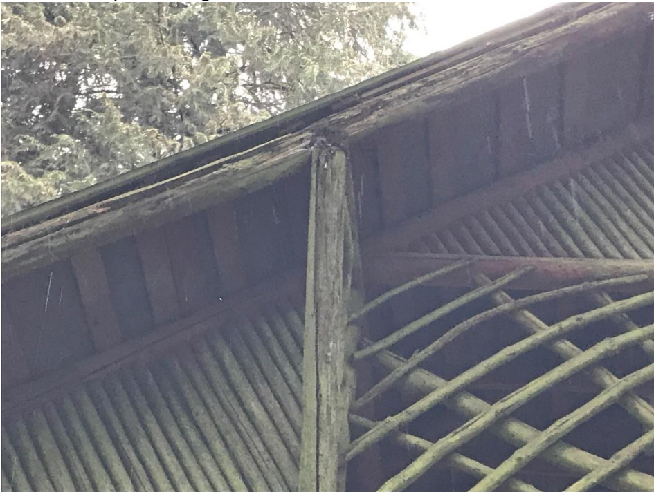
Picture 6 – dry rot damage
