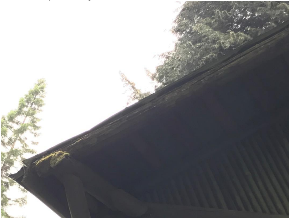
Picture 8 – dry rot damage
