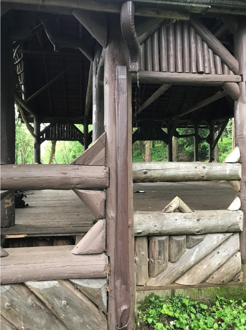
Picture 11 – damaged downspout
