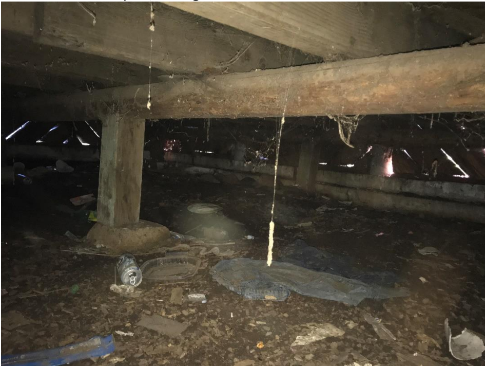
Picture 13 – shifted post/footing
