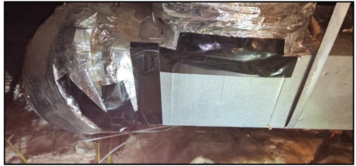
44. Ductwork repaired with improper duct tape
