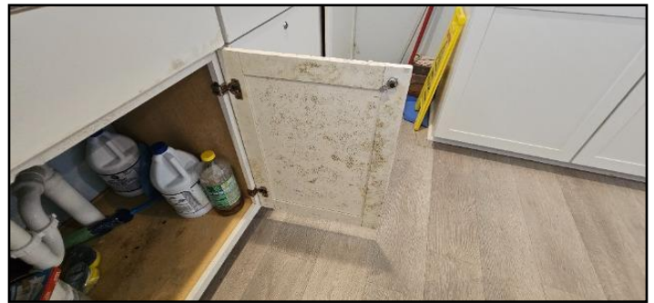
26. Visible growth on cabinets
