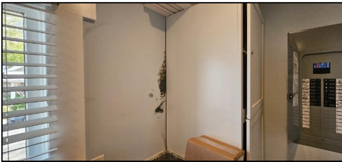
25. Visible growth on wall behind cabinet
