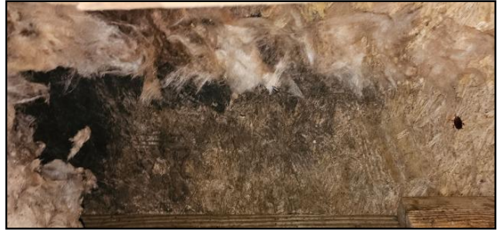
73. Visible mold growth
