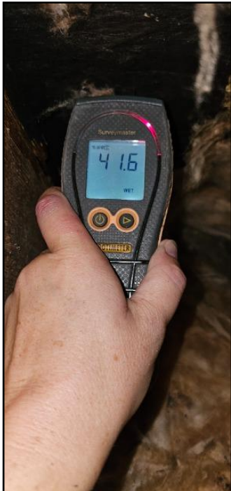
76. Wet subfloor near HVAC plenum
