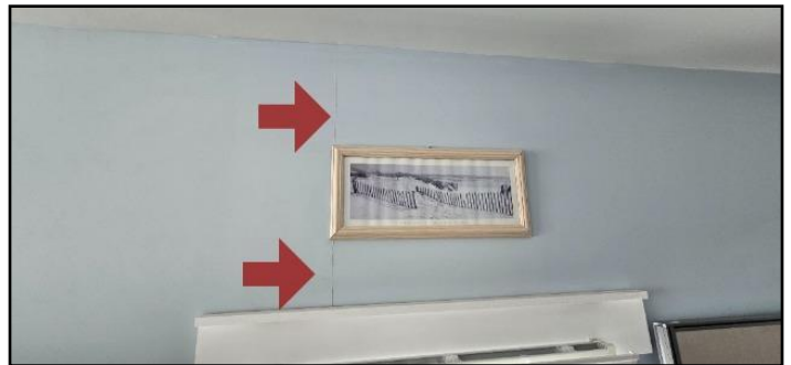
10. Crack in drywall
