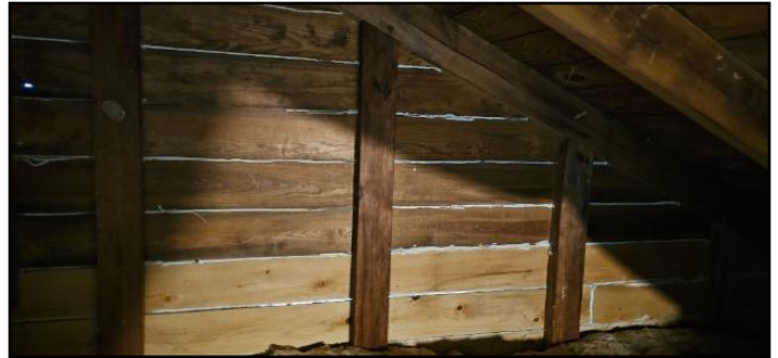
38. Gaps between wood siding
