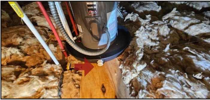
43. Drain line capped - improper
