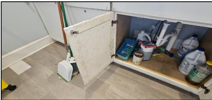
27. Visible growth on cabinets
