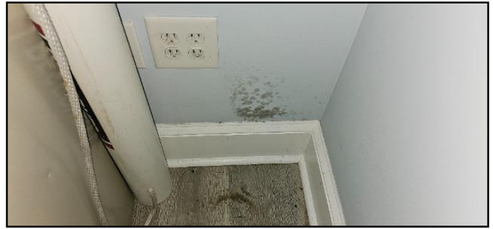
22. Visible growth on drywall near plenum
