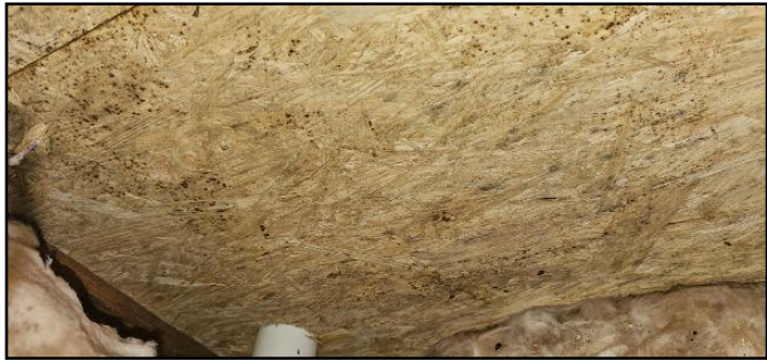
81. Visible growth on subfloor
