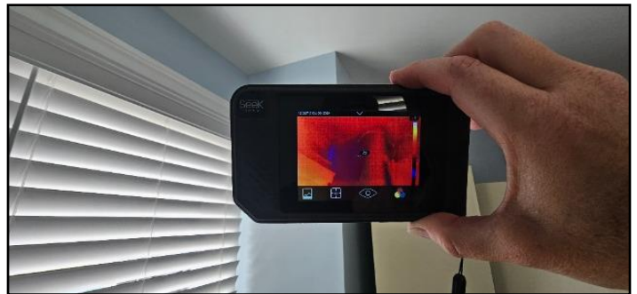
18. Moisture noted at drywall around plenum
