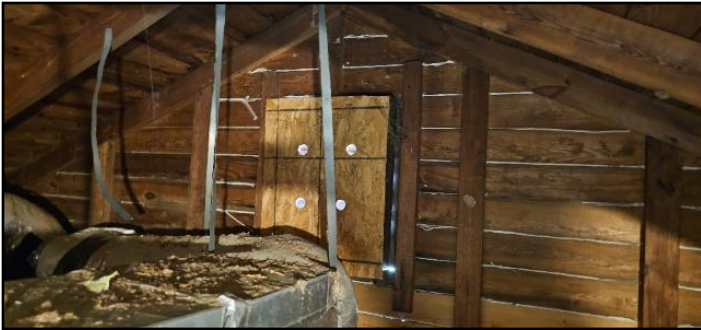
37. Gable vent covered with plywood
