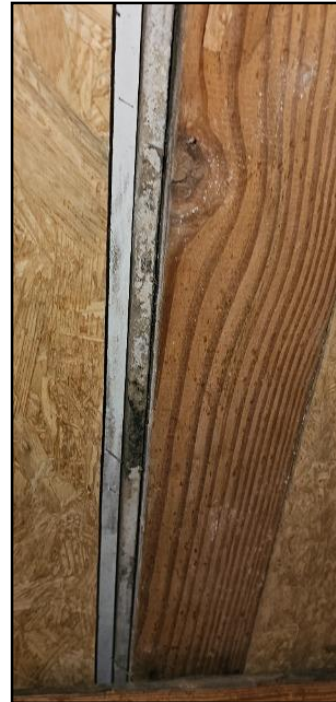
65. Microbial growth on drywall
