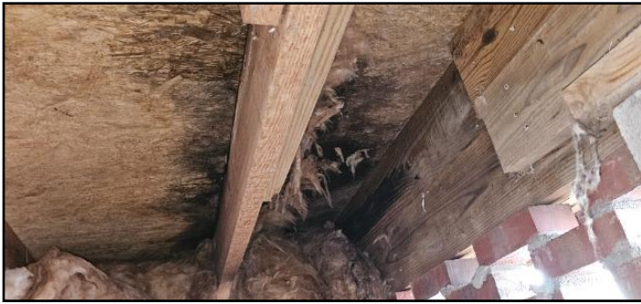
80. Water damaged subfloor
