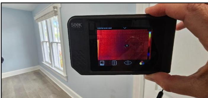
31. Moistuer in wall beside window
