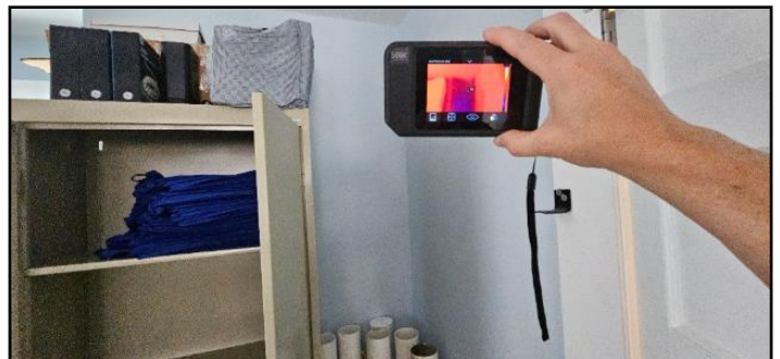
20. Moisture noted at drywall around plenum
