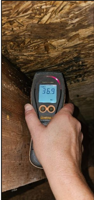
72. Wet subfloor near HVAC plenum
