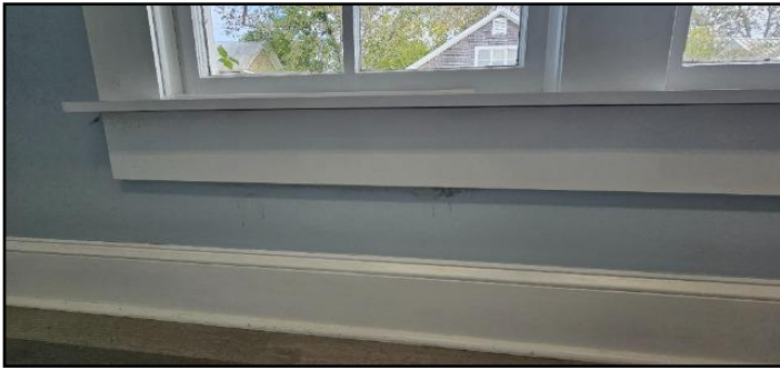
5. Visible growth or infiltration below window
