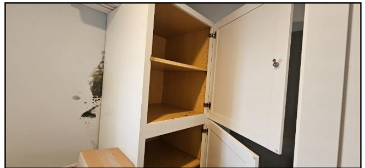
28. Visible growth on cabinets
