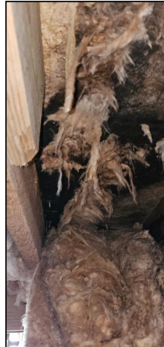
75. Visible mold growth on subfloor
