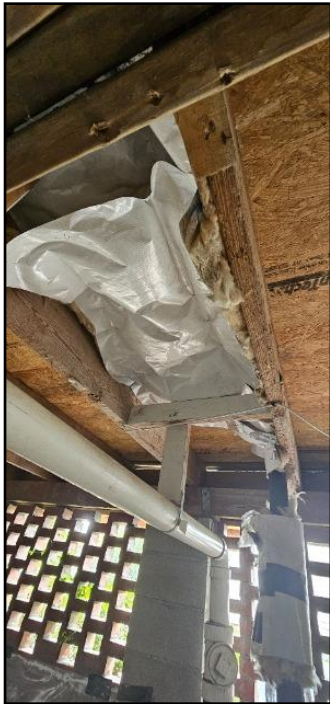
66. Plumbing access limited due to plastic
