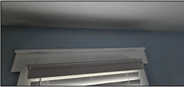
13. Visible growth above window
