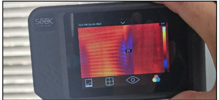
16. Moisture noted around window
