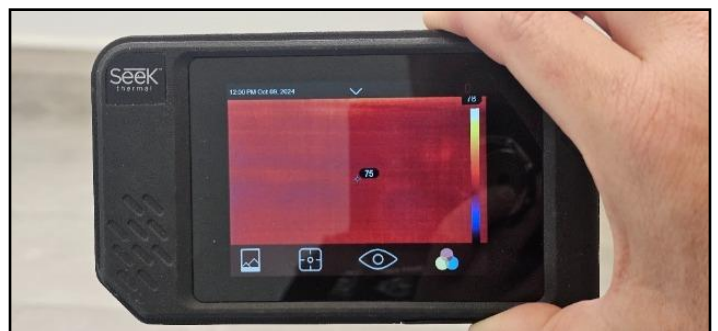
32. Moisture in wall above baseboards
