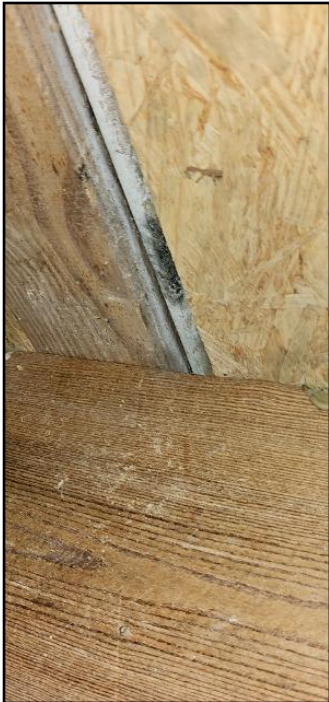
64. Microbial growth on drywall
