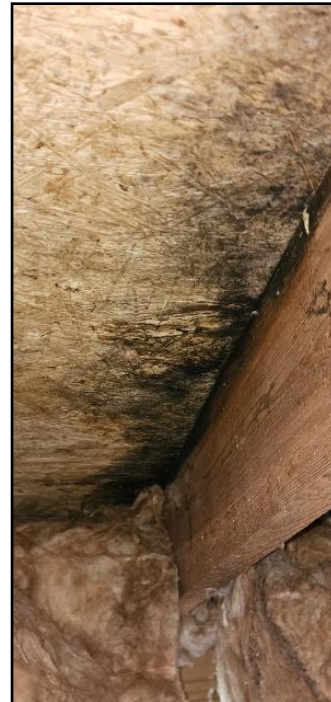
77. Wet subfloor near HVAC plenum
