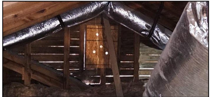
42. Gaps in siding - no wall sheathing installed
