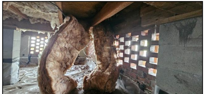
79. Area of wet subfloor due to condensation HVAC
