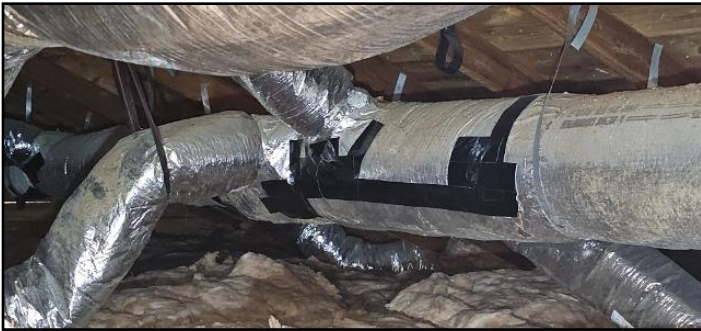
45. Ductwork repaired with improper duct tape
