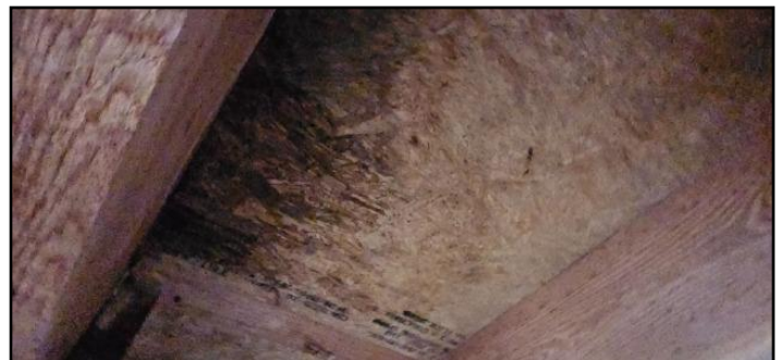
71. Wet subfloor near HVAC plenum
