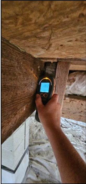
62. Wet drywall exposed in crawlspace
