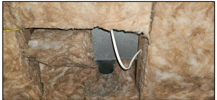
40. Exhaust fan not exhausted to exterior
