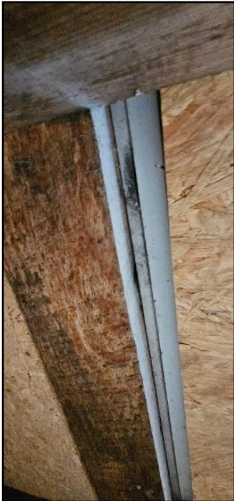
60. Microbial growth on drywall exposed in crawl
