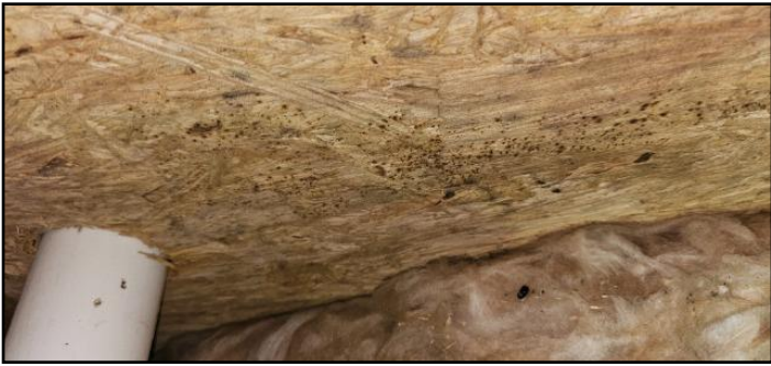
82. Visible growth on subfloor
