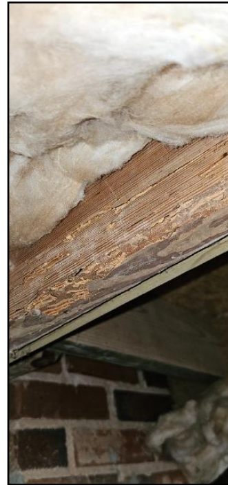
67. Visible growth on floor joists
