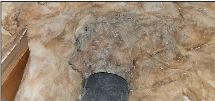
41. Discolored insulation should be removed
