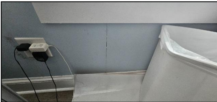
9. Visible growth at baseboard
