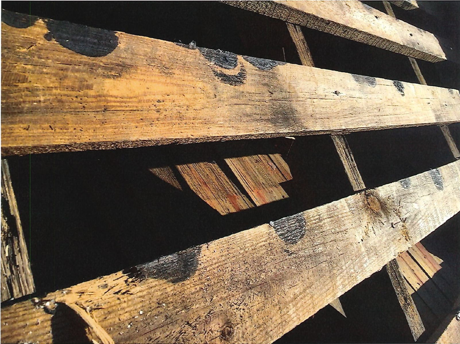
View of Top of Porch Roof Sheathing with original cedar shake shingles underneath on portion of main roof
