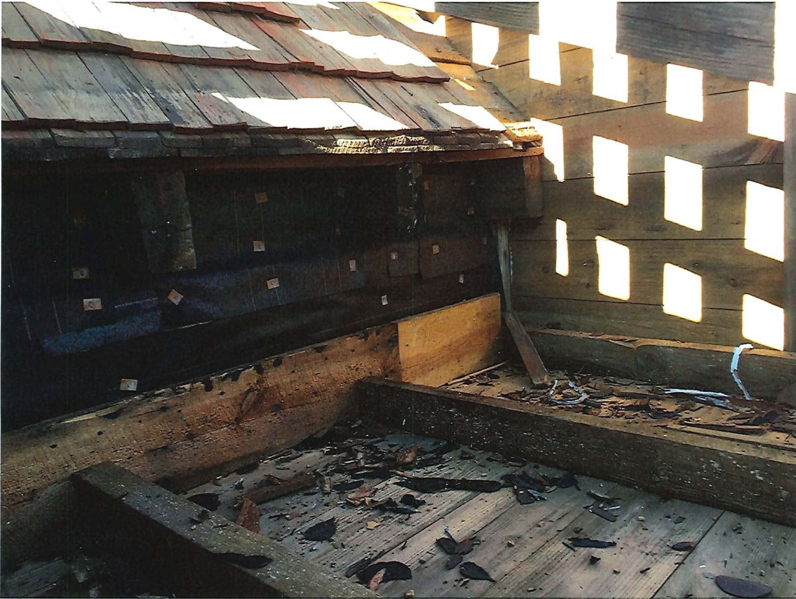
View under porch roof's tie to main roof (looking to side facing Main Street) with original framing and original cedar shake shingles
