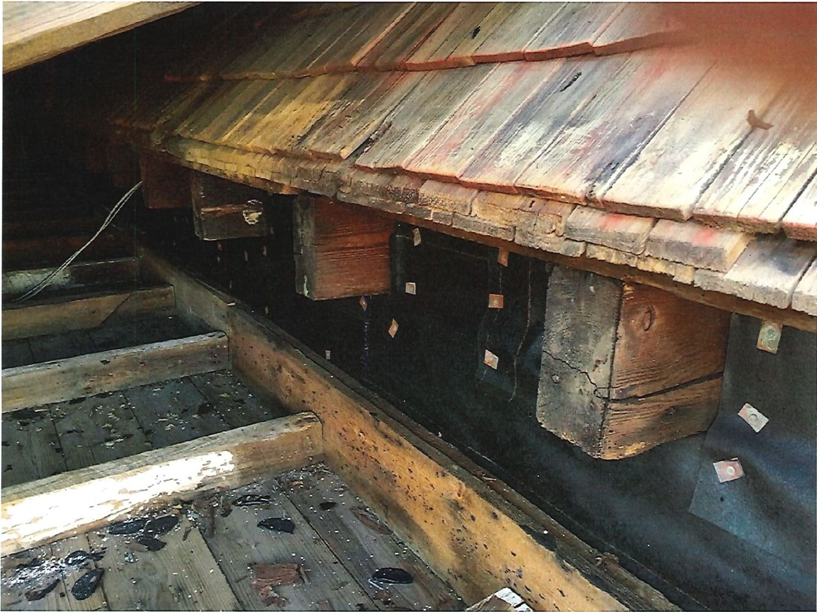
Zoom in view under porch roof's tie to main roof with original framing and original cedar shake shingles
