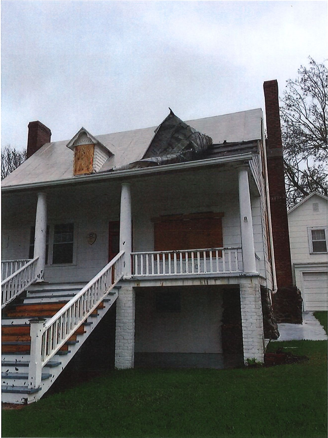
Porch roof damage from hurricane Florence 2018
