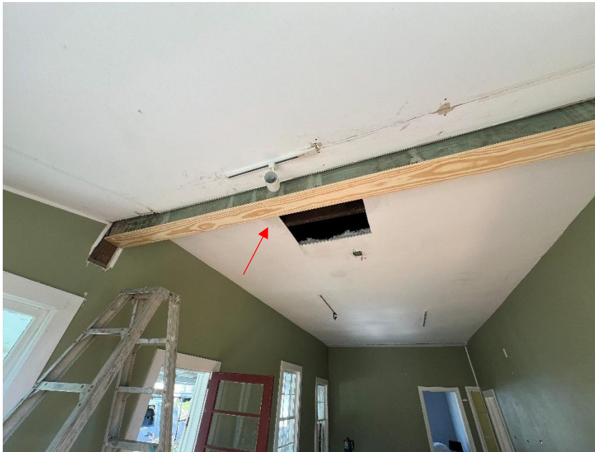
Exposed beam shows original house color
