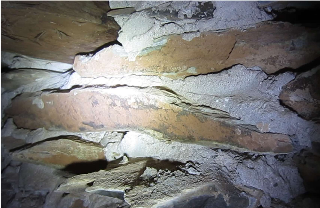
Figure 12 – Foundation Stacked Stone - Moisture affected mortar strength
