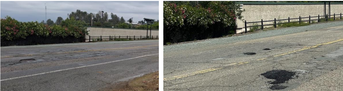
Ridge Road (Pothole first notice and fixed)
