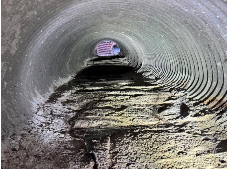
Storm drain under Gopher Flat Rd. the top of the pipe is intact.
