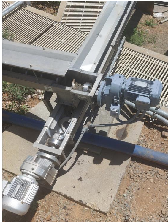
New Gear box for Headworks Auger
