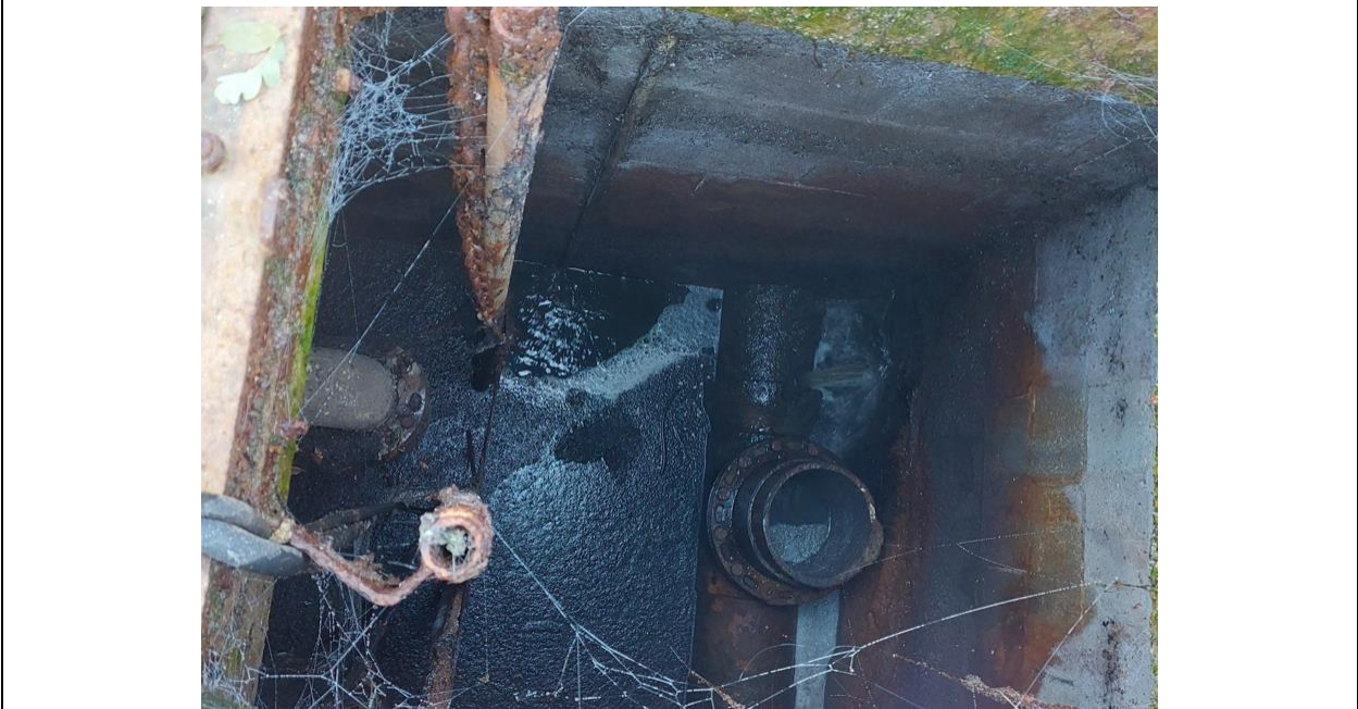
Return Valve in E-pump Vault
