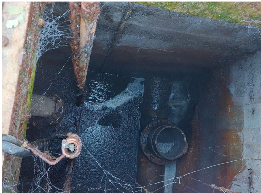
Return Valve in E-pump Vault
