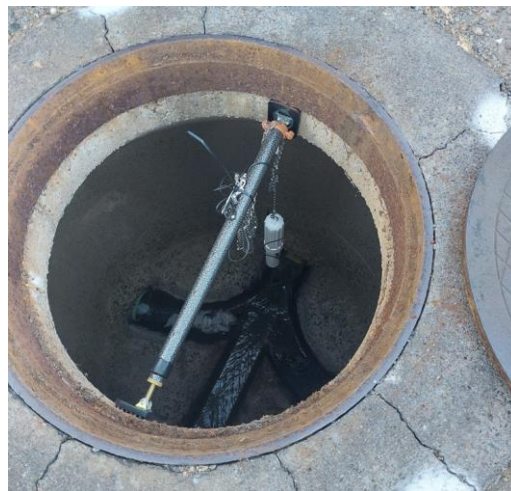
Flow Meter Installation-Complete
