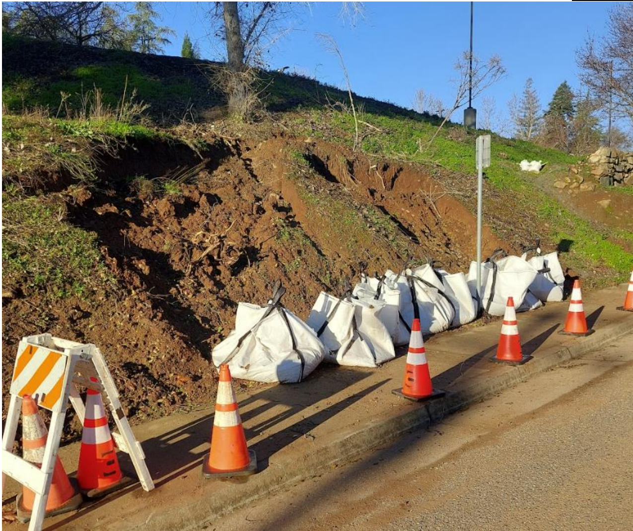
(Sidewalk Left closed on Dec 20th as precautionary measure until hillside can be stabilized)
