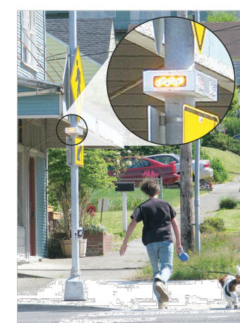
RRFB with Pedestrian Verification Light
