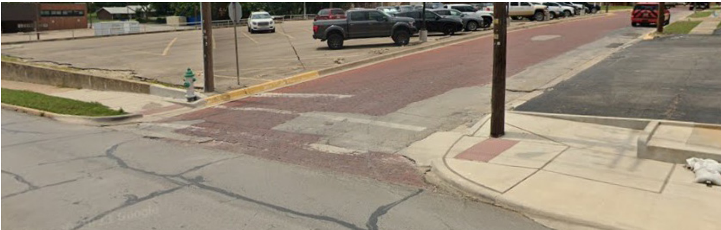
Example of sidewalk with uneven surfaces and limited ADA accessibility (corner of Washington & Barton Avenues)
