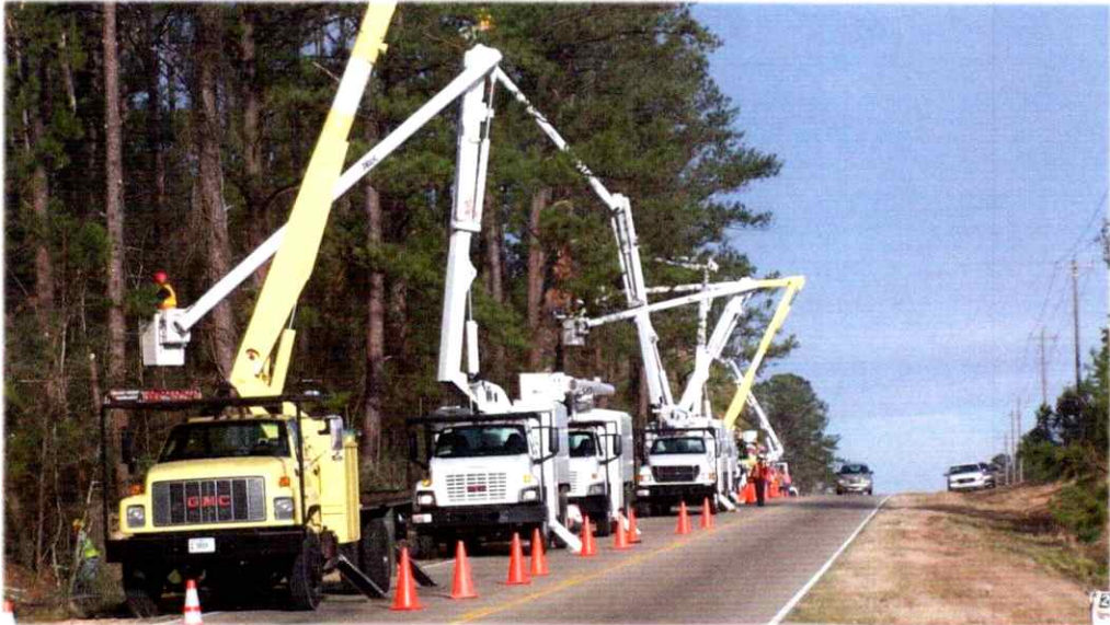
Hazard Tree Removal (Leaner)
