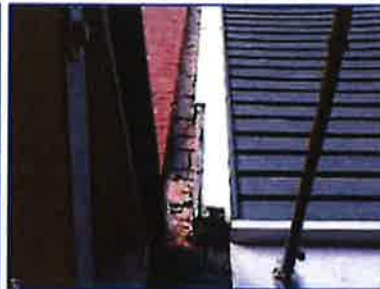
Areas of damaged/missing trim at front of building
