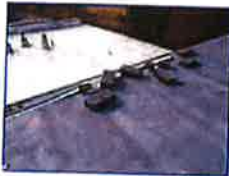
Debris on roof
