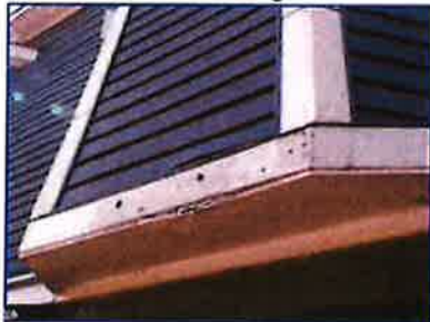
Areas of damaged trim at front of building
