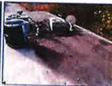
Ponding on flat roof
