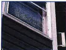
Areas of damaged window at front of building
