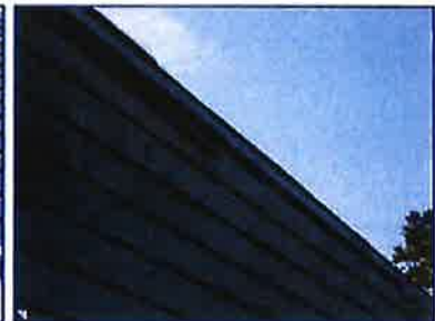
Areas of damaged/missing trim at right side of building
