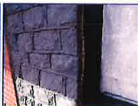
Areas of open joints around window frames
