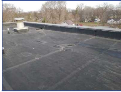
SECTION B - Def 3 - Before Photo
