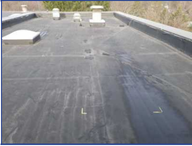
SECTION B - Def 3 - Before Photo
