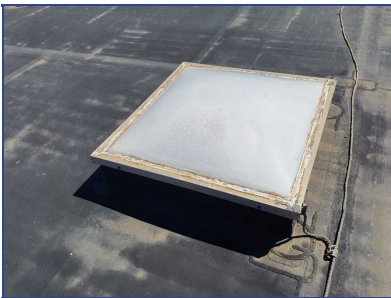
Skylight Safety Awareness
