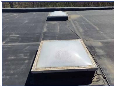
Skylight Safety Awareness
