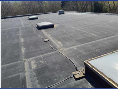
Skylight Safety Awareness
