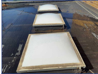
Skylight Safety Awareness
