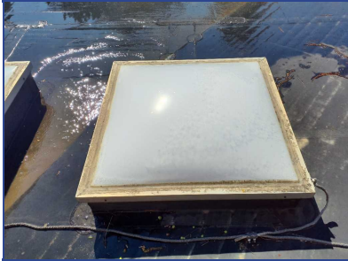
Skylight Safety Awareness
