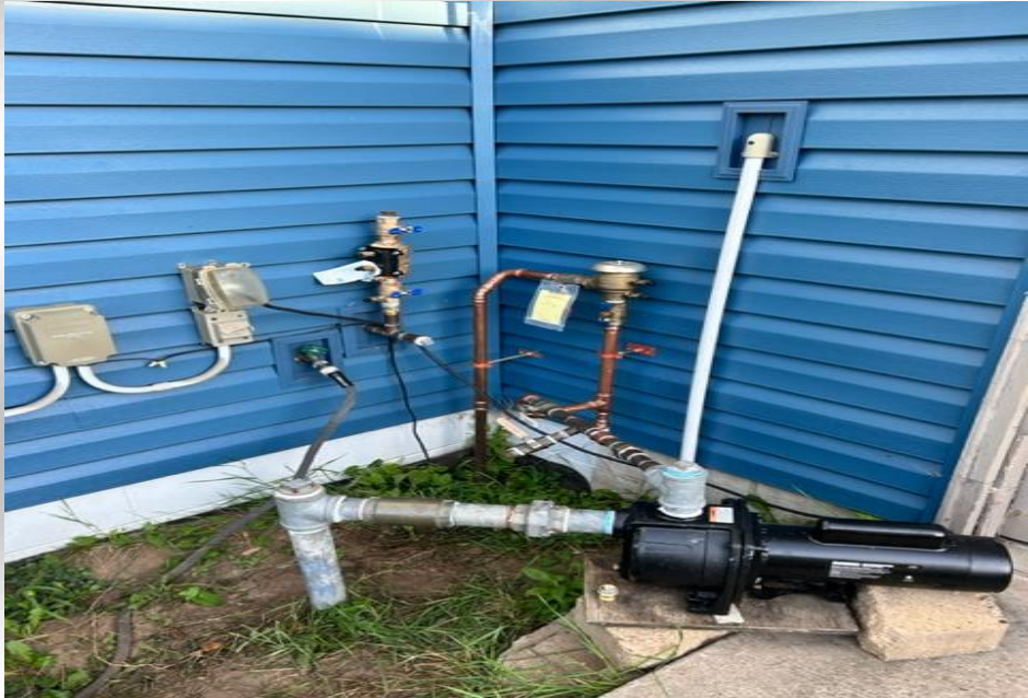
After contacting the homeowner, the necessary repair was made to correct the issue.
