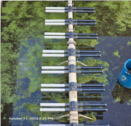
The picture to the right is the diffusers with the membranes installed and diffusers without.
