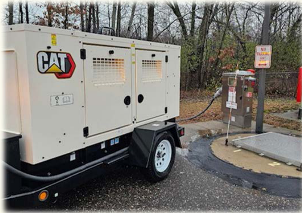
Photo: Generator successfully tested at one of our lift stations, demonstrating full operational capability.
