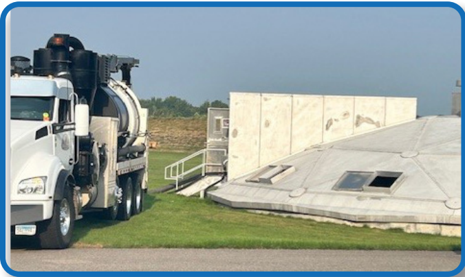
David's hydro-vac assisted cleaning the bottom of the clarifier with their vac truck.
