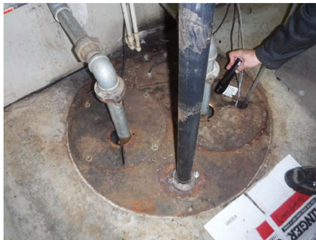
Figure 1. Sampling location for the Waterfront Building. Sump is located below the metal cover. Metal pipes shown are sump pump discharge lines, and plastic pipe is an influent drain line.
