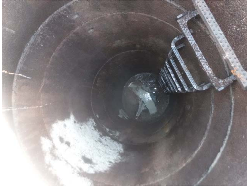
Figure 4. Skamania Lodge discharge manhole sampling location.
