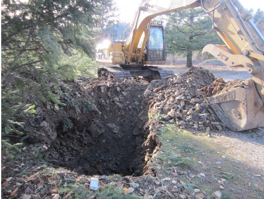
Photograph 7: Excavation TP9, which had angular cobble fill from surface to approximately 5 feet below ground surface. Photograph taken facing south.
