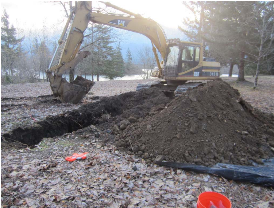
Photograph 3: Excavation TP2 along the eastern foundation of the large building. Photograph taken facing south.
