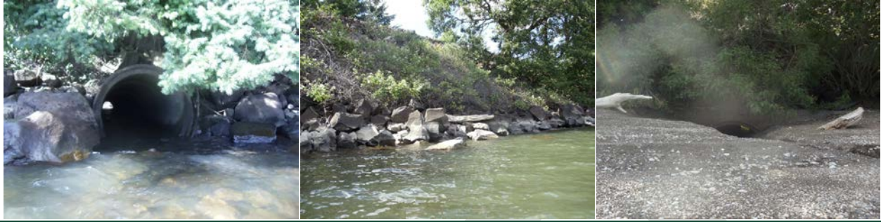
Columbia River Reach 1 Degradation & Restoration Opportunities Differing culvert sizes & elevations, Riprap slopes, and Invasive species along the SR 14/BNSF railroad berm Photo Credits: Ben Shumaker (2013).
