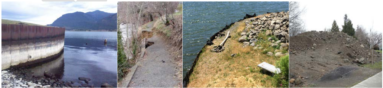
Columbia River Reach 2 Degradation & Restoration Opportunities Sheetpile, active erosion, and staging along the Port of Skamania's Stevenson Shoreline Restoration & Enhancement Project Photo Credits: John McSherry (2010, 2012), Ben Shumaker (2015, 2018).
