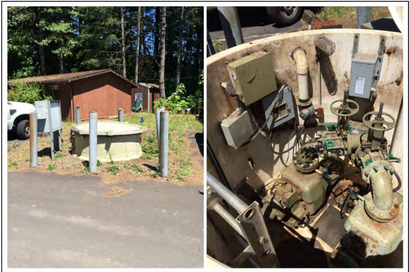
Figure 3-5. Fairgrounds Pump Station Photos
