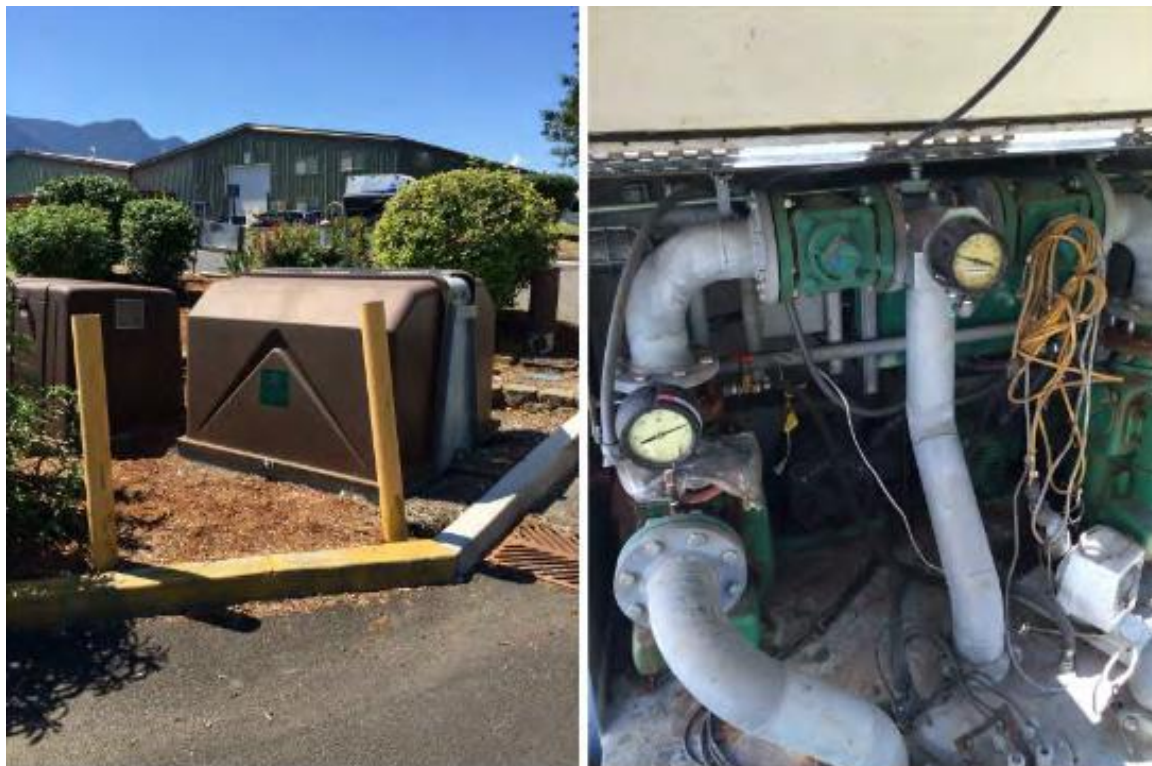
Figure 2-3 Kanaka Creek Pump Station Photos
