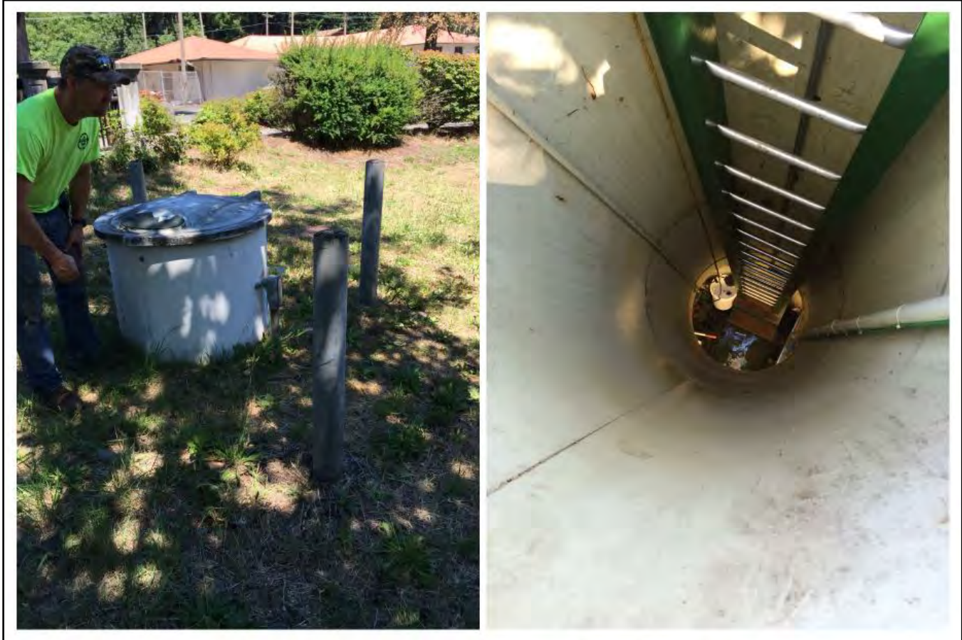
Figure 3-4. Rock Creek Pump Station Photos
