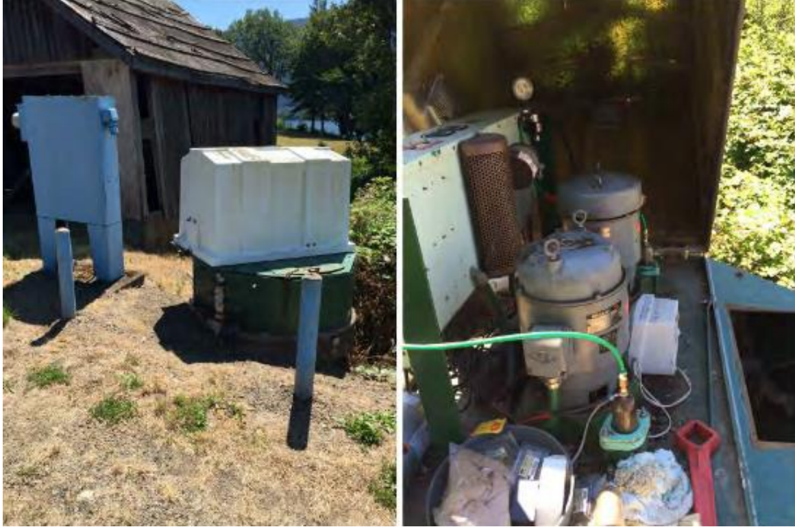
Figure 2-2 Cascade Pump Station Photos
