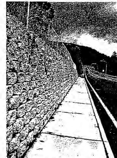
Not Appropriate: Keystone block retaining walls
