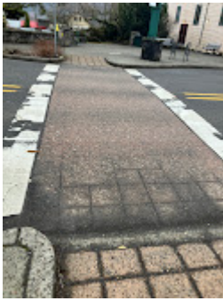
Degraded crosswalk markings nr. Walnut Park.jpg 5828K
