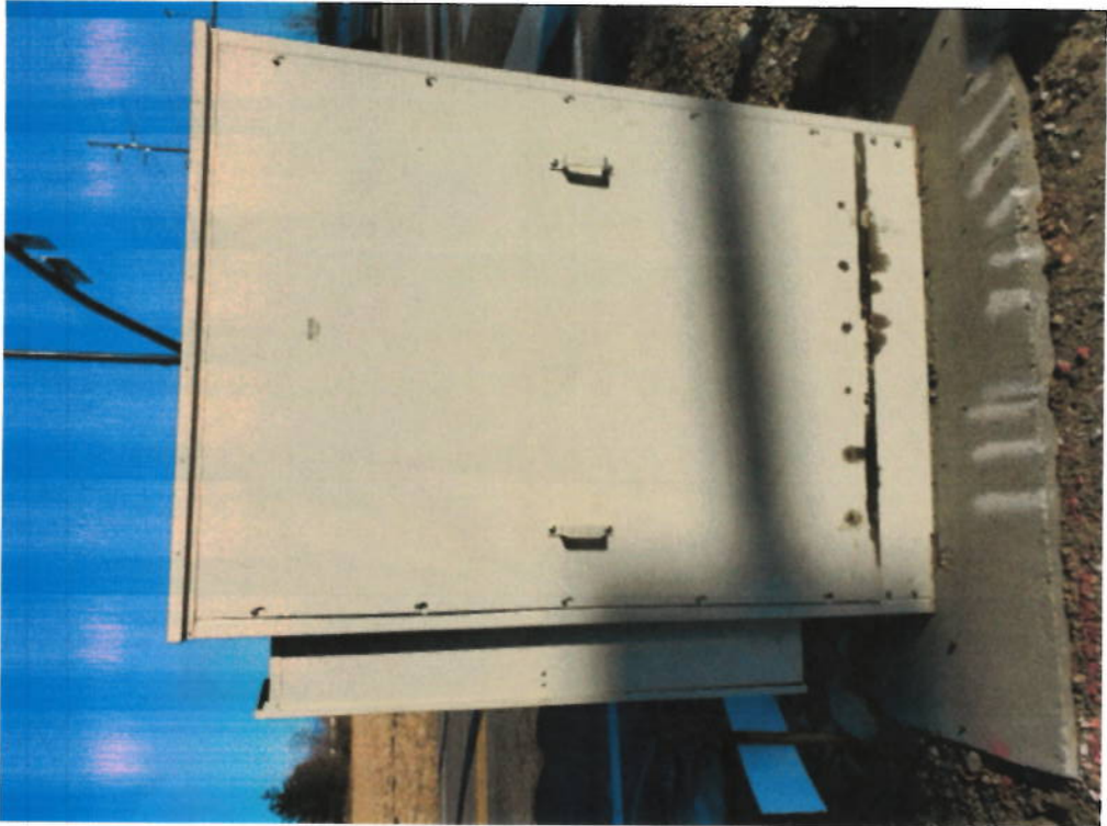
Pic #1/3 Toon Town – Main box – back (next to street outside of sidewalk on Plummer) 67' H x 48' W x 16.5 W (3) pictures of this utility box included
