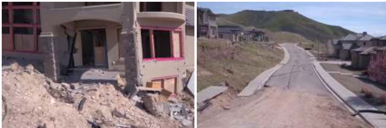
Figure 16-2. Residential and Infrastructure Damage, Alto Via Court
