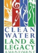
Stabilized bank on Rice Creek includes riprap at the bottom of the slope and native seed, shrub stakes, and erosion control blanket at the top of the slope.
