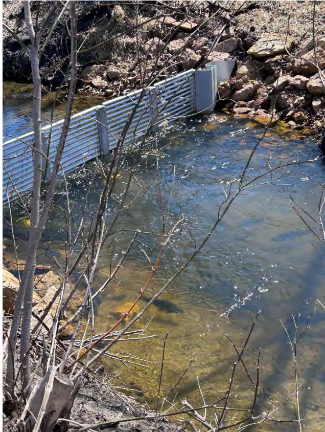
Figure 6 Johanna Creek Carp Barrier at New Brighton Community Center in New Brighton, MN
