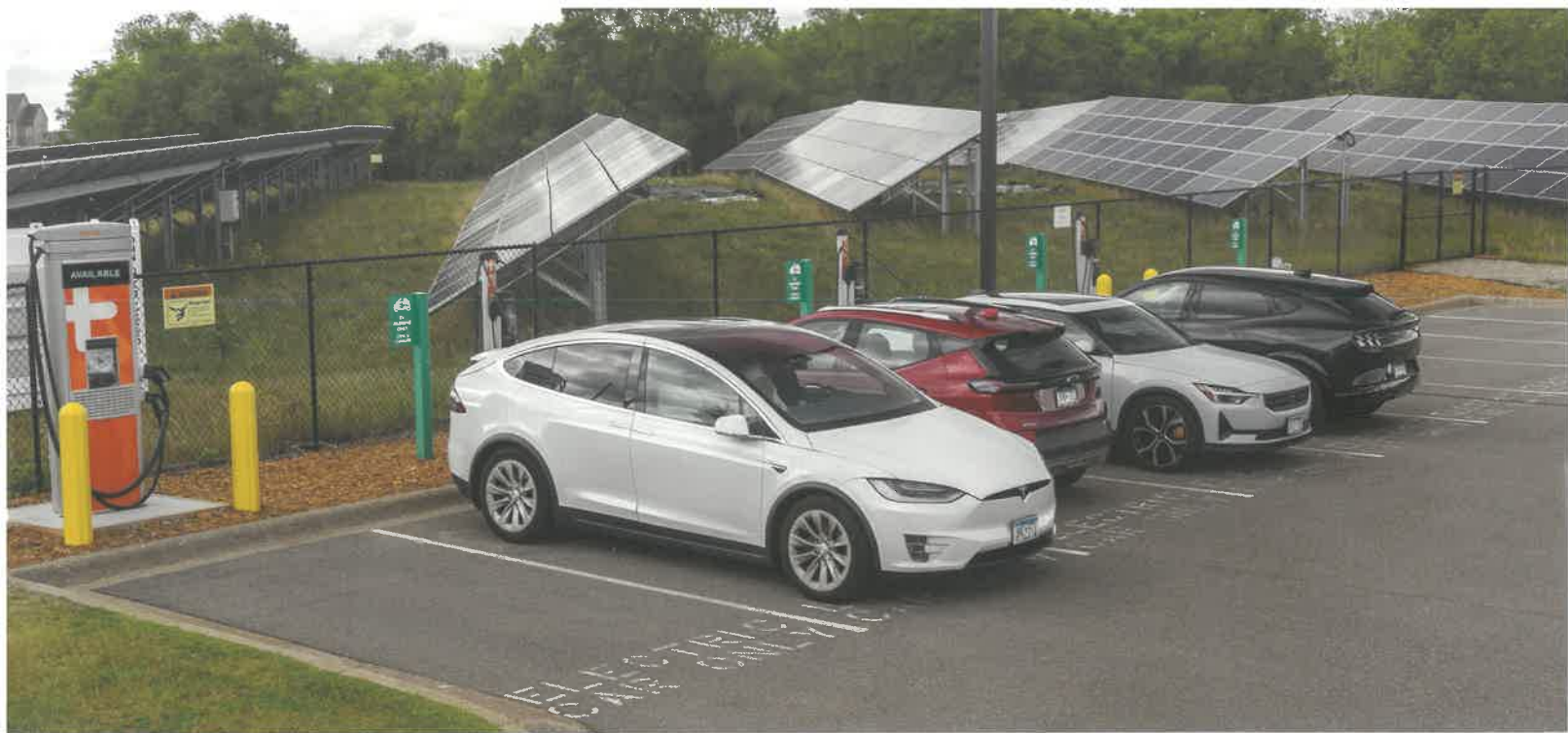
EV owners can access three ChargePoint Level 2 charging stations and one DC fast charging station next to the community solar garden at our headquarters in Ramsey.
