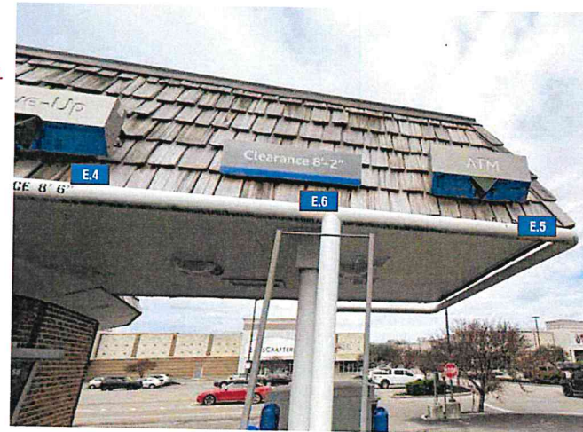
EAST DRIVE-UP ELEVATION SCALE: 3/32" = 1'-0" - EXISTING DU-B, DU-C AND TC-CL-W TO BE REMOVED AND RE-INSTALLED
