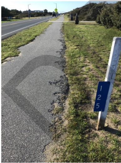
Figure E – Raveling of asphalt edges
