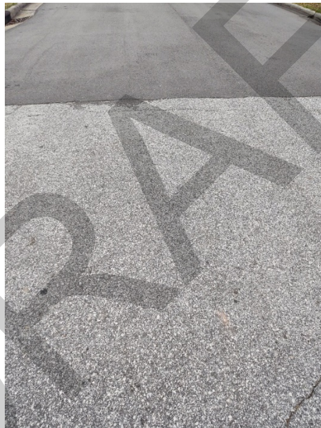
Figure 9: Oxidation versus newer pavement (top of picture)
