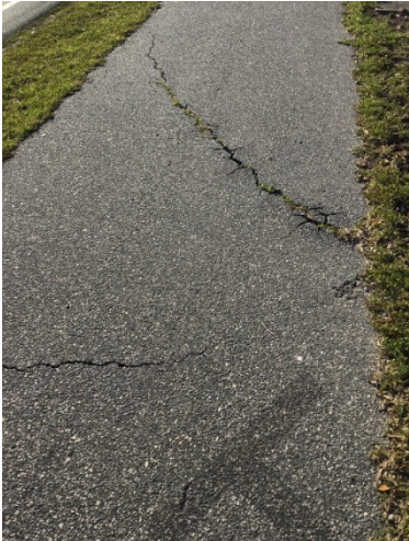
Figure D – More cracking due to roots
