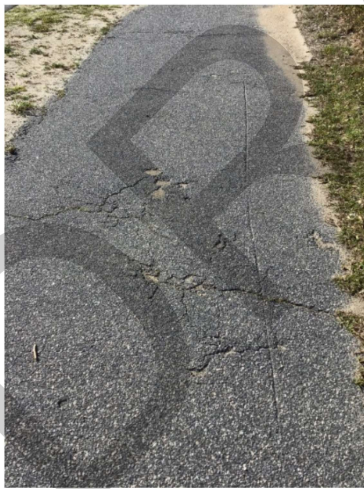
Figure A - Transverse Cracking
