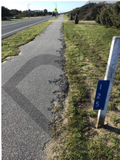
Figure E – Raveling of asphalt edges
