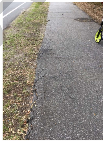
Figure B – Edge Cracking
