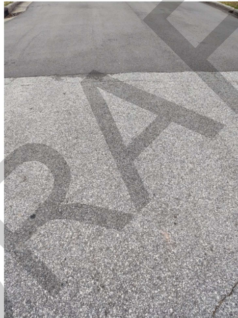
Figure 9: Oxidation versus newer pavement (top of picture)
