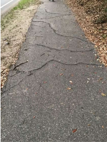
Figure C – Root intrusion cracks
