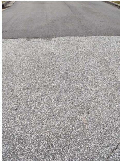
Figure 9: Oxidation versus newer pavement (top of picture)
