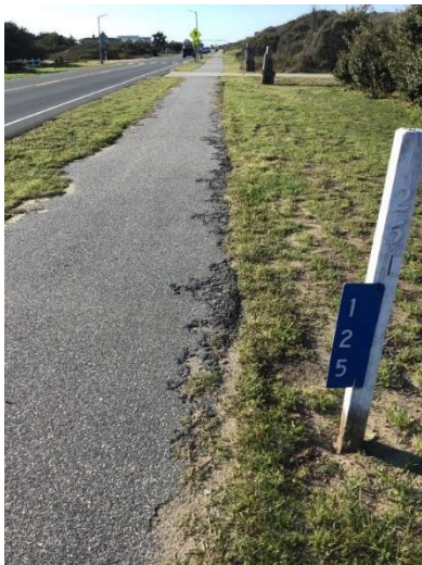
Figure E – Raveling of asphalt edges
