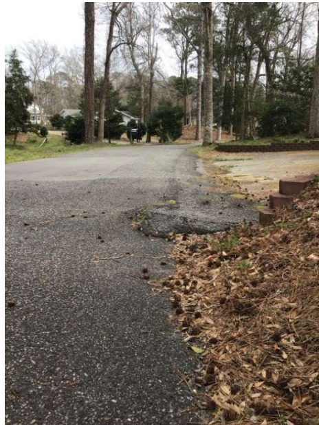
Figure 10: Tree roots affecting ride quality on E. Holly Trail
