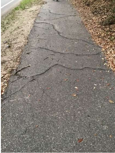
Figure C – Root intrusion cracks
