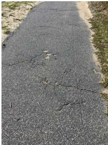
Figure A - Transverse Cracking
