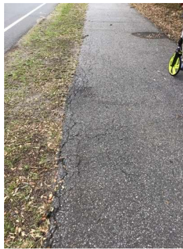
Figure B – Edge Cracking
